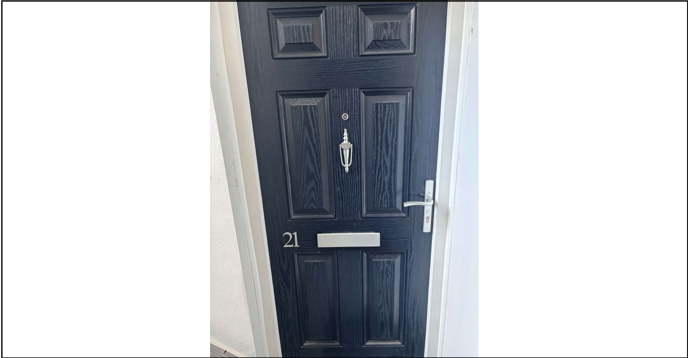
Photo No. 5 Every Flat Door replaced January 2024 all have internal self closer
