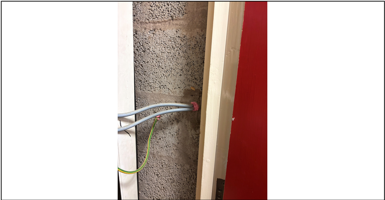
Photo No. 3 Compartmentation breaches in service cupboard between a & b
