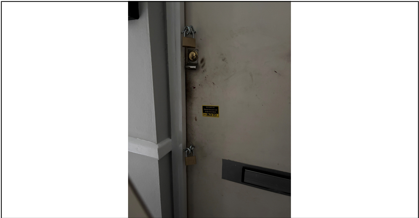
Photo No. 4 Door to 109e damaged
