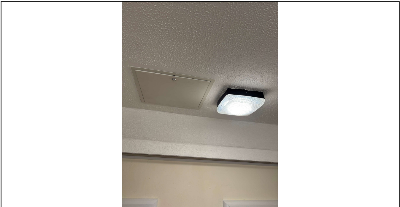
Photo No. 4 Top Floor which has no smoke lobby, Fire resistant loft hatch Maintained EML.
