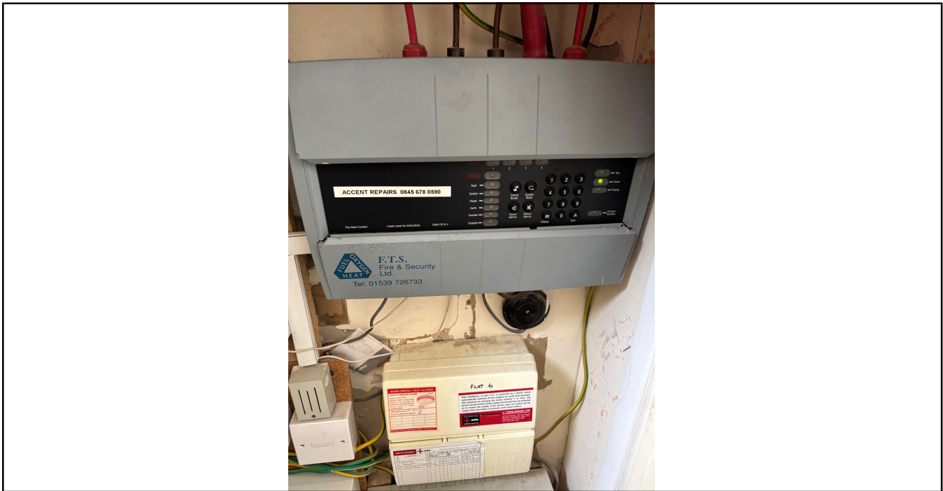
Photo No. 4 Fire panel showing no faults
