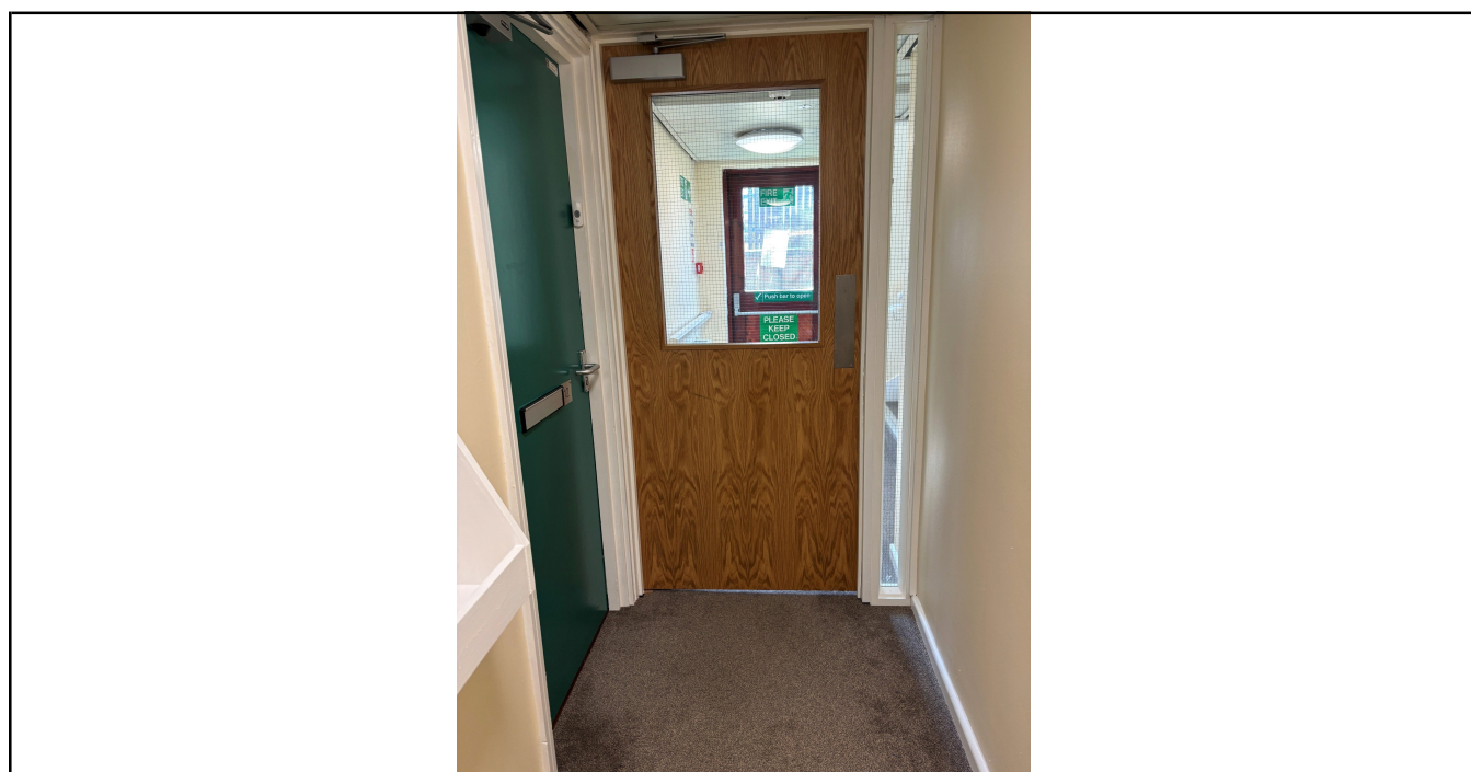
Photo No. 6 Large gap under staircase door nr Flat 12
