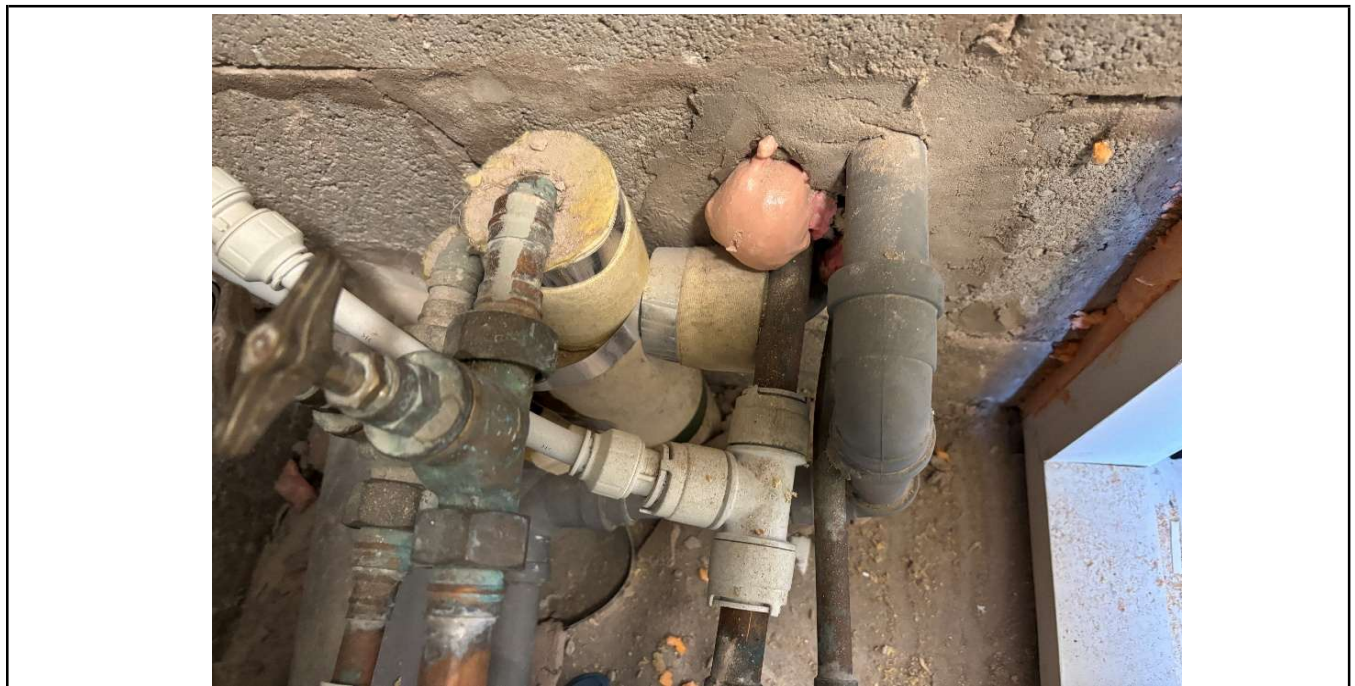
Photo No. 3 Example of breach of compartment in service cupboard
