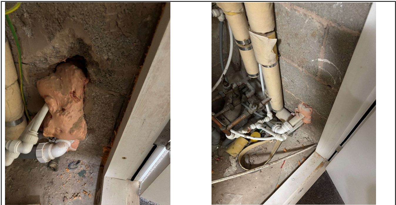
Photo No. 2 Examples of compartment breaches in service cupboard.
