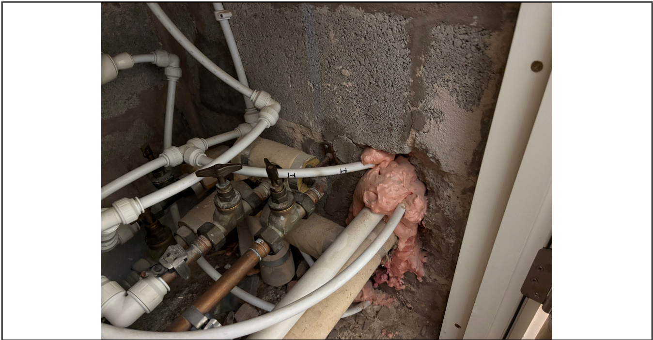
Photo No. 1 Example of compartment breache in service cupboard
