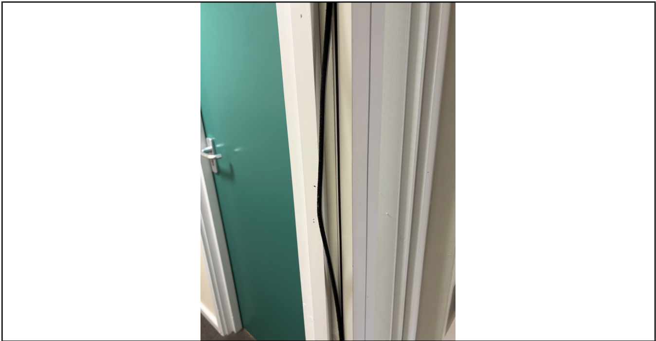
Photo No. 7 Combined seal damaged - Corridor door nr guest flat
