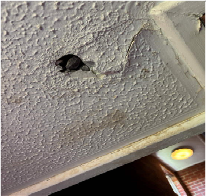
Photo No. 6 Compartmentation breach in Ground floor ceiling
