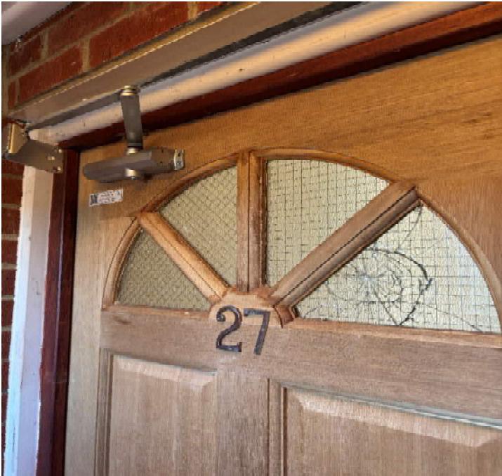
Photo No. 5 Broken glass panel in door 27
