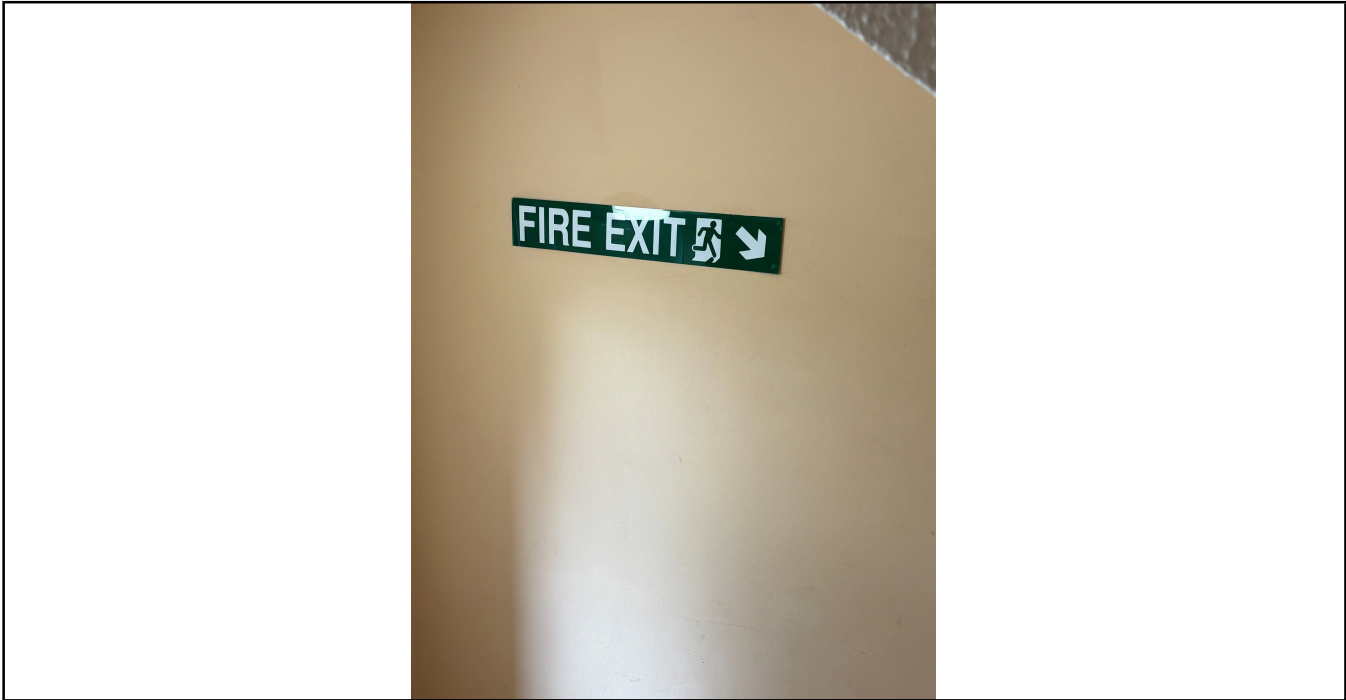
Photo No. 5 Directional Exit signage
