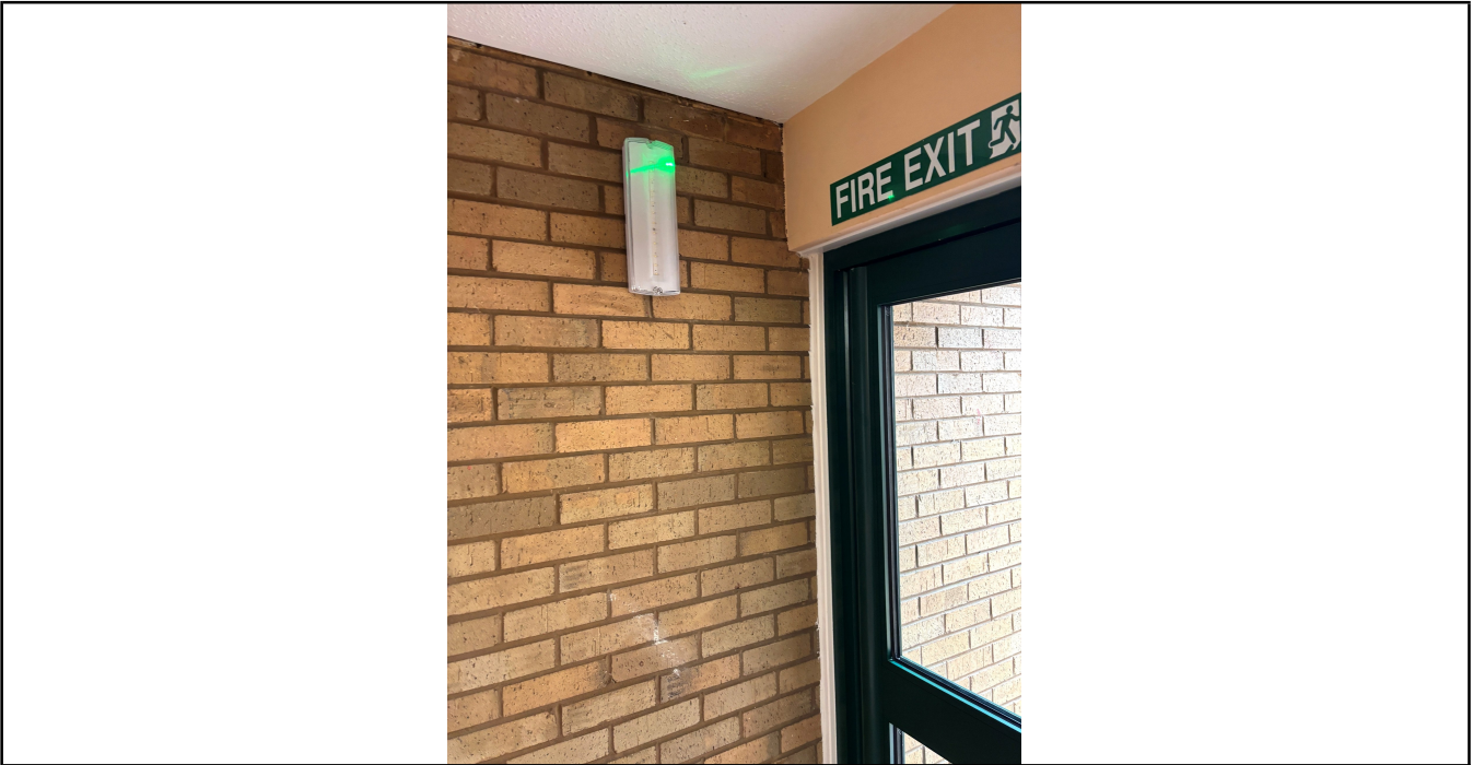
Photo No. 3 Emergency Lighting
