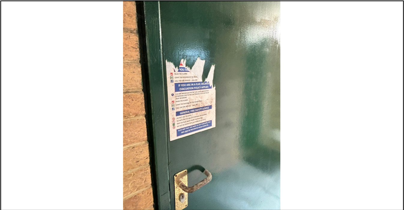
Photo No. 2 Fire evacuation notice torn - Replaced
