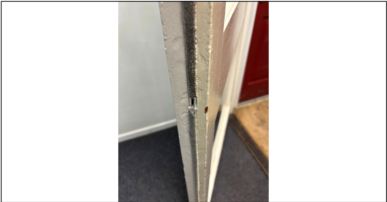
Photo No. 2 Smoke seal damaged on lobby door into Flats a-b
