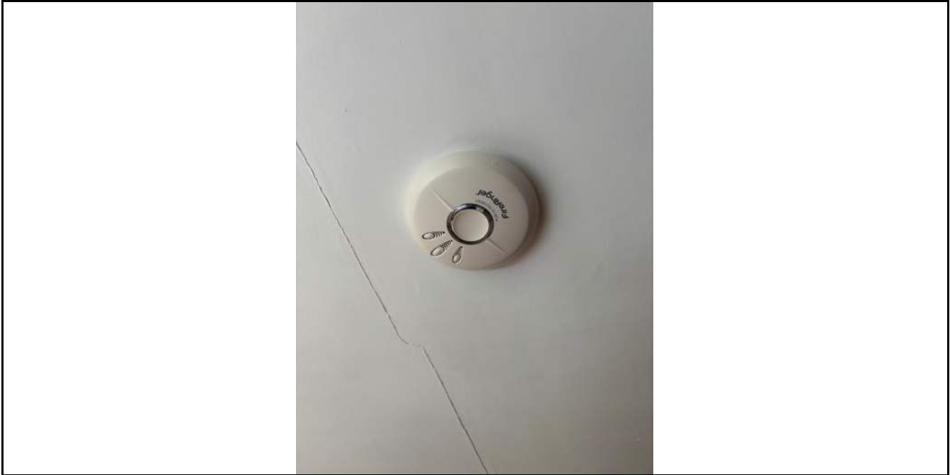
Photo No. 1 Smoke detector fitted F2 with batteries removed
