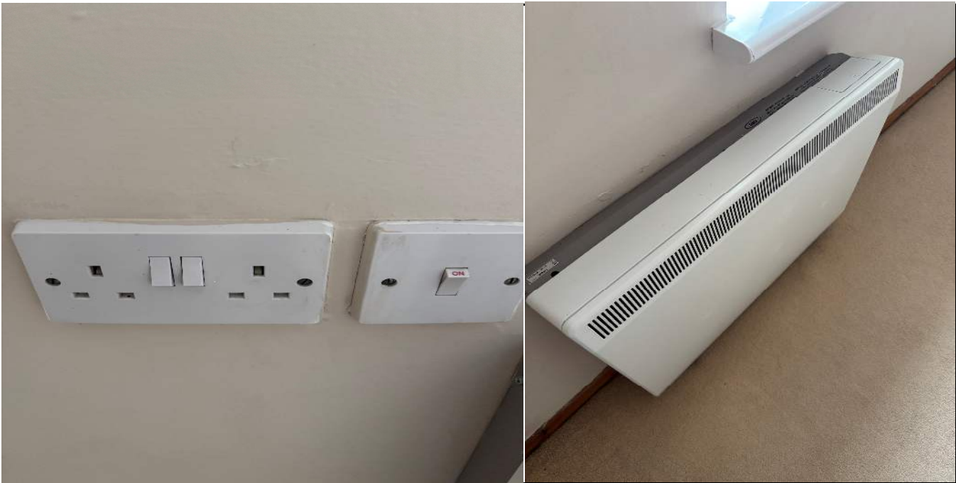
Photo No. 3 Electrical appliances in good condition and secured
