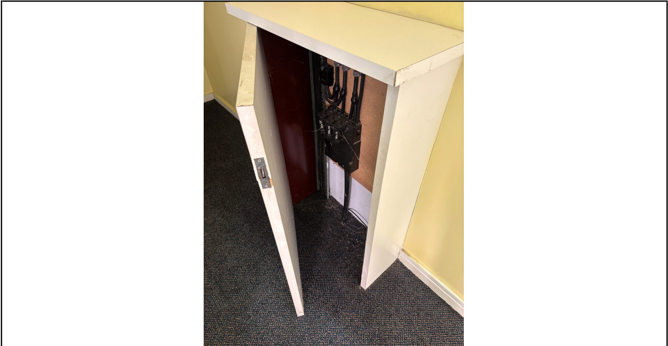
Photo No. 11 The electrical intake cupboard in the rear stairwell requires replacing.
