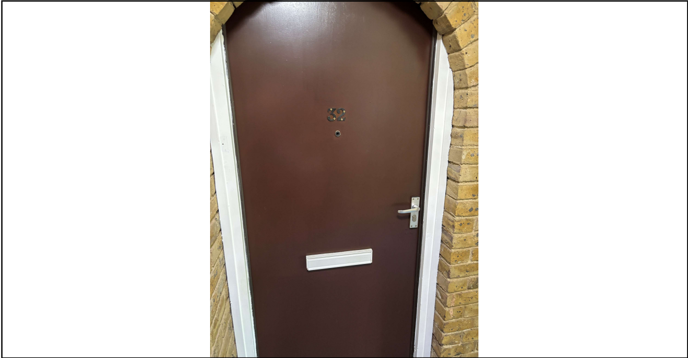
Photo No. 7 Standar Flat Door self closers internal due to design. All Flat Doors Replaced 2024.
