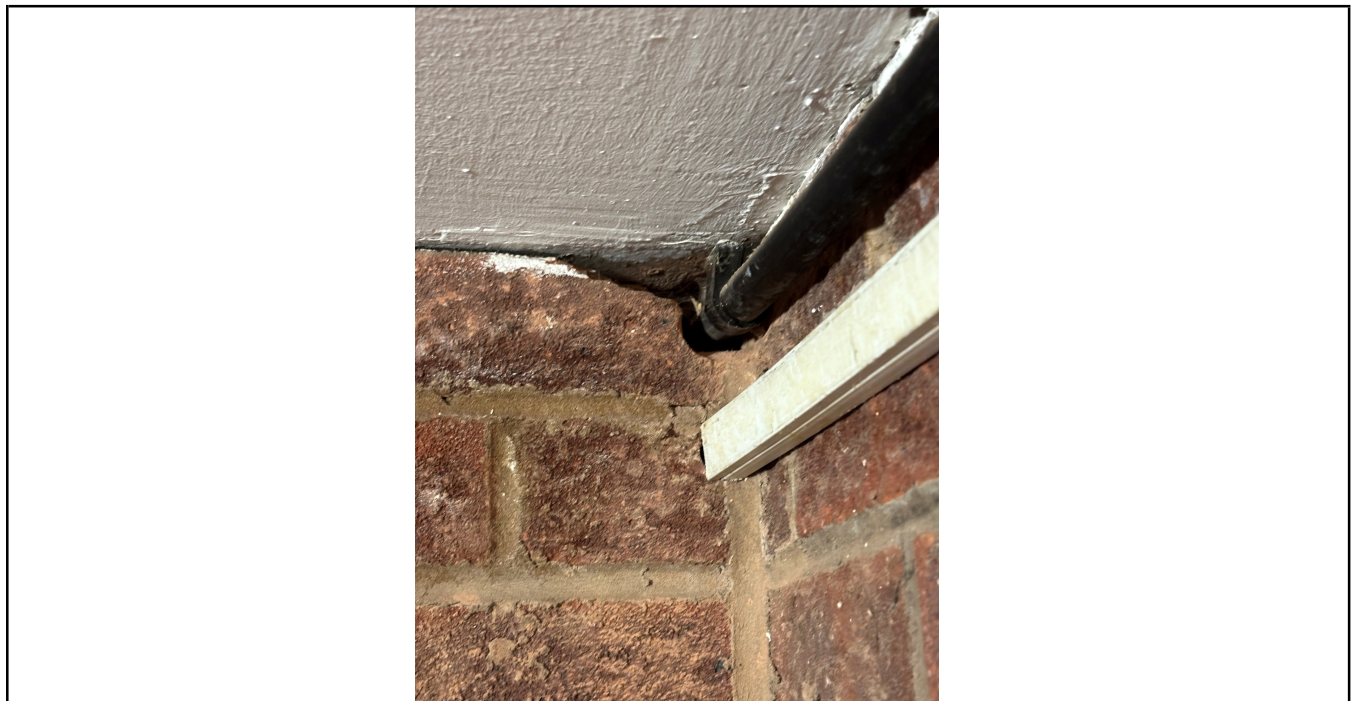
Photo No. 1 Breach of compartmentation from electrical room
