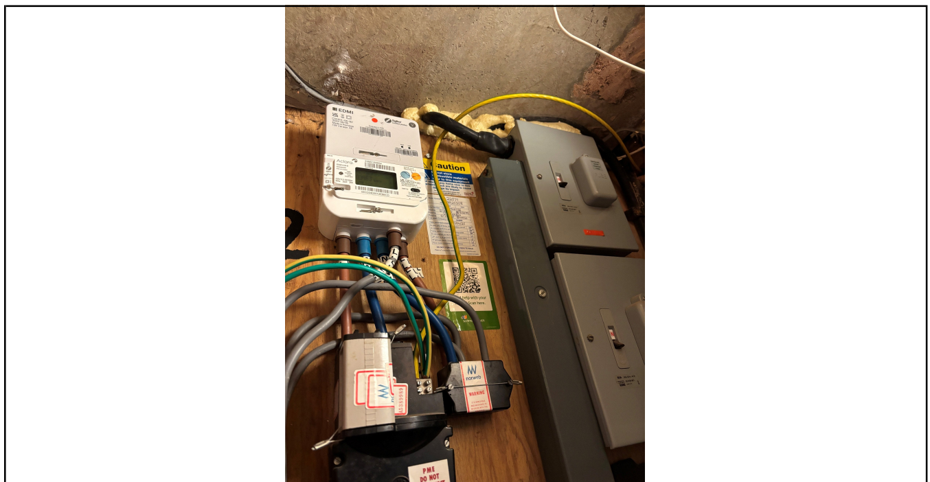
Photo No. 2 Yellow expanding foam used to seal compartment breaches GroundF
