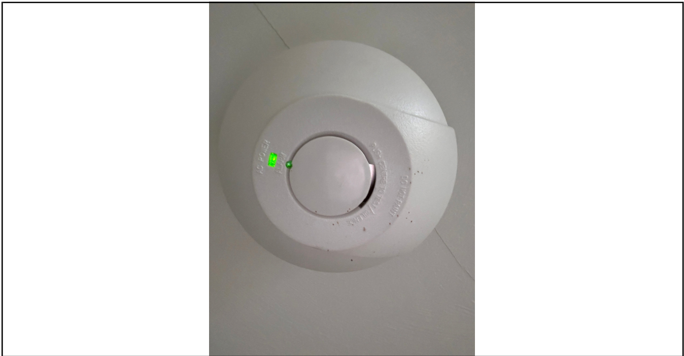
Photo No. 4 Smoke detection in communal area
