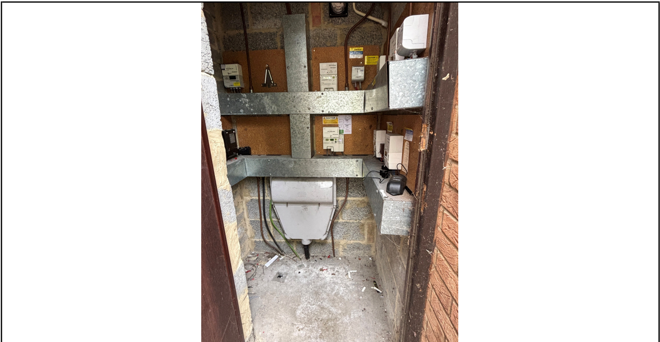
Photo No. 4 The electrical cupboard was clear at the time of the audit.
