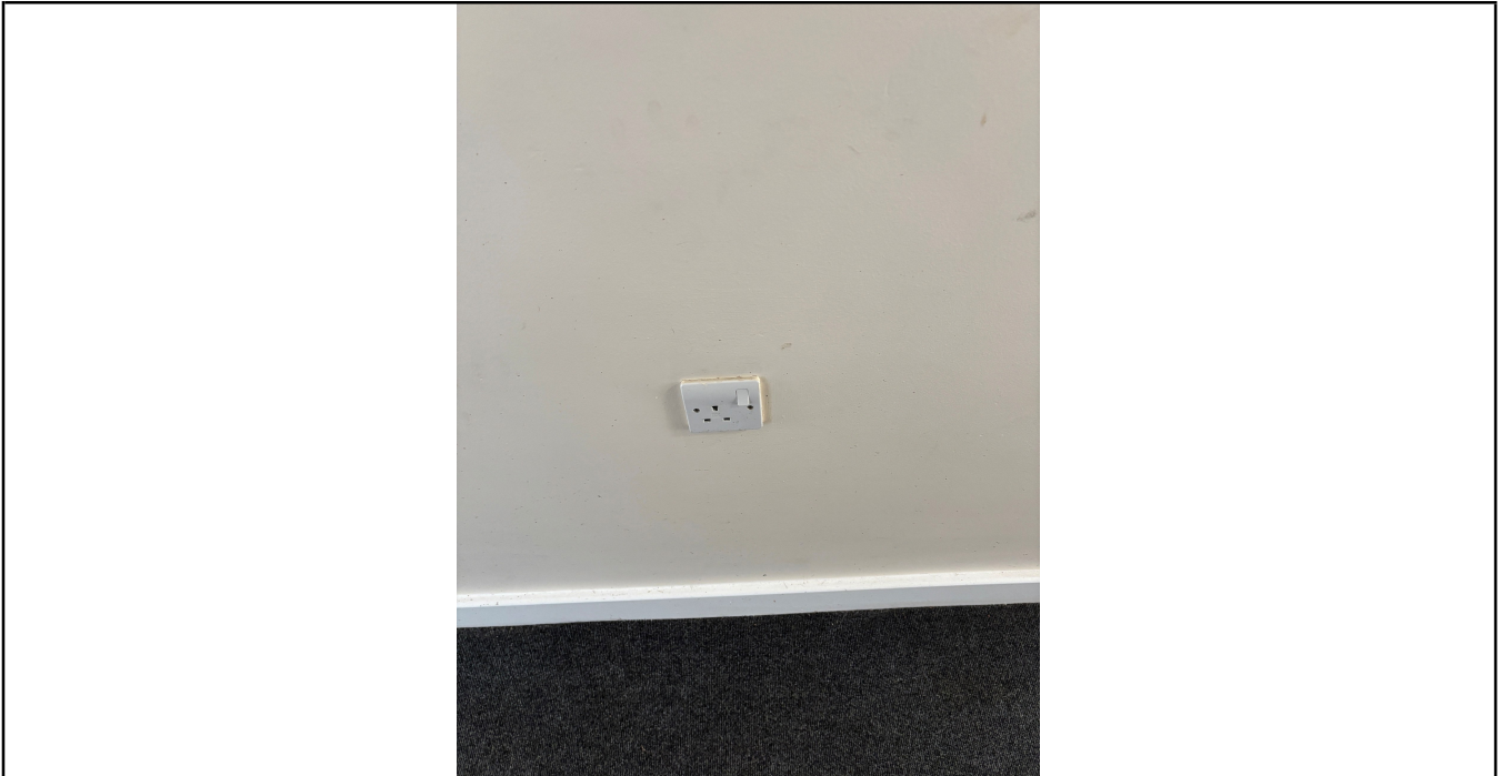
Photo No. 7 Sockets need to be lockable due to battery charging in the communal area
