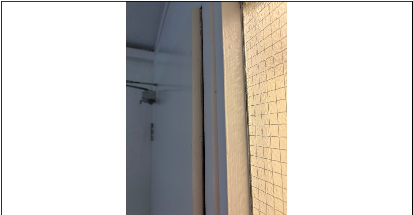
Photo No. 1 Fire door not fully self closing into lobby a-b
