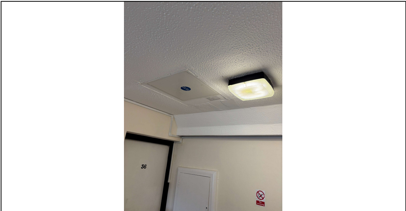
Photo No. 4 Top floor No Smoke lobby, Fire resisting loft Hatch Maintained EML system.
