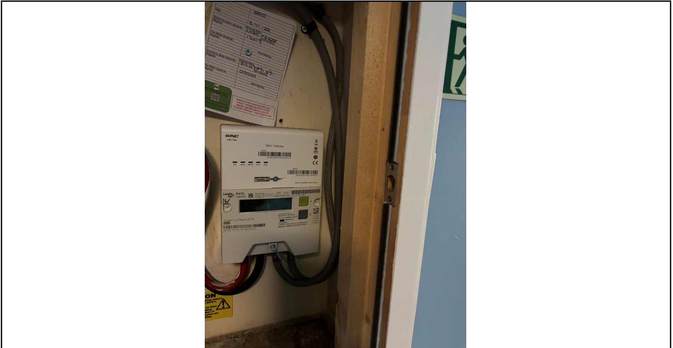
Photo No. 7 All electrical intake cupboard checked were clear of rubbish and Fire stopp
