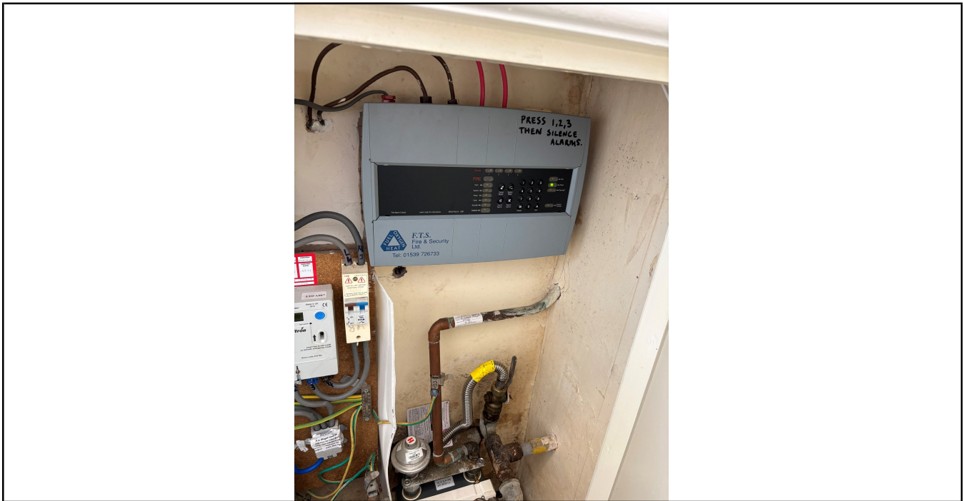
Photo No. 2 Fire alarm panel showing no faults
