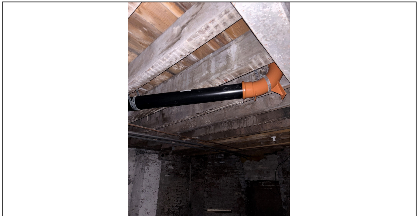
Photo No. 5 Basement has no fire separation
