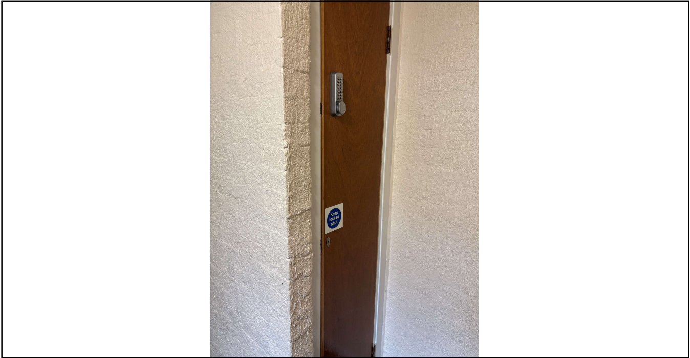
Photo No. 1 Electric cupboard door on each floor.
