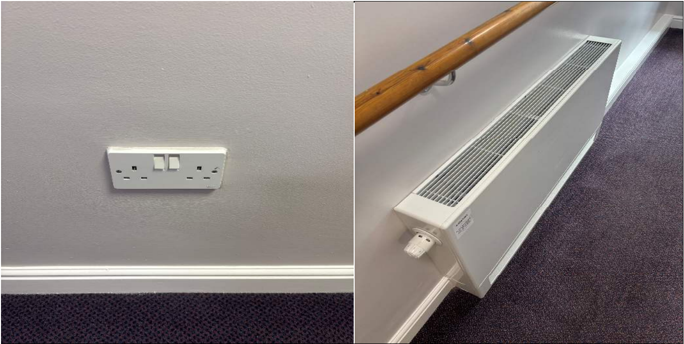
Photo No. 12 Electrical fittings in good condition
