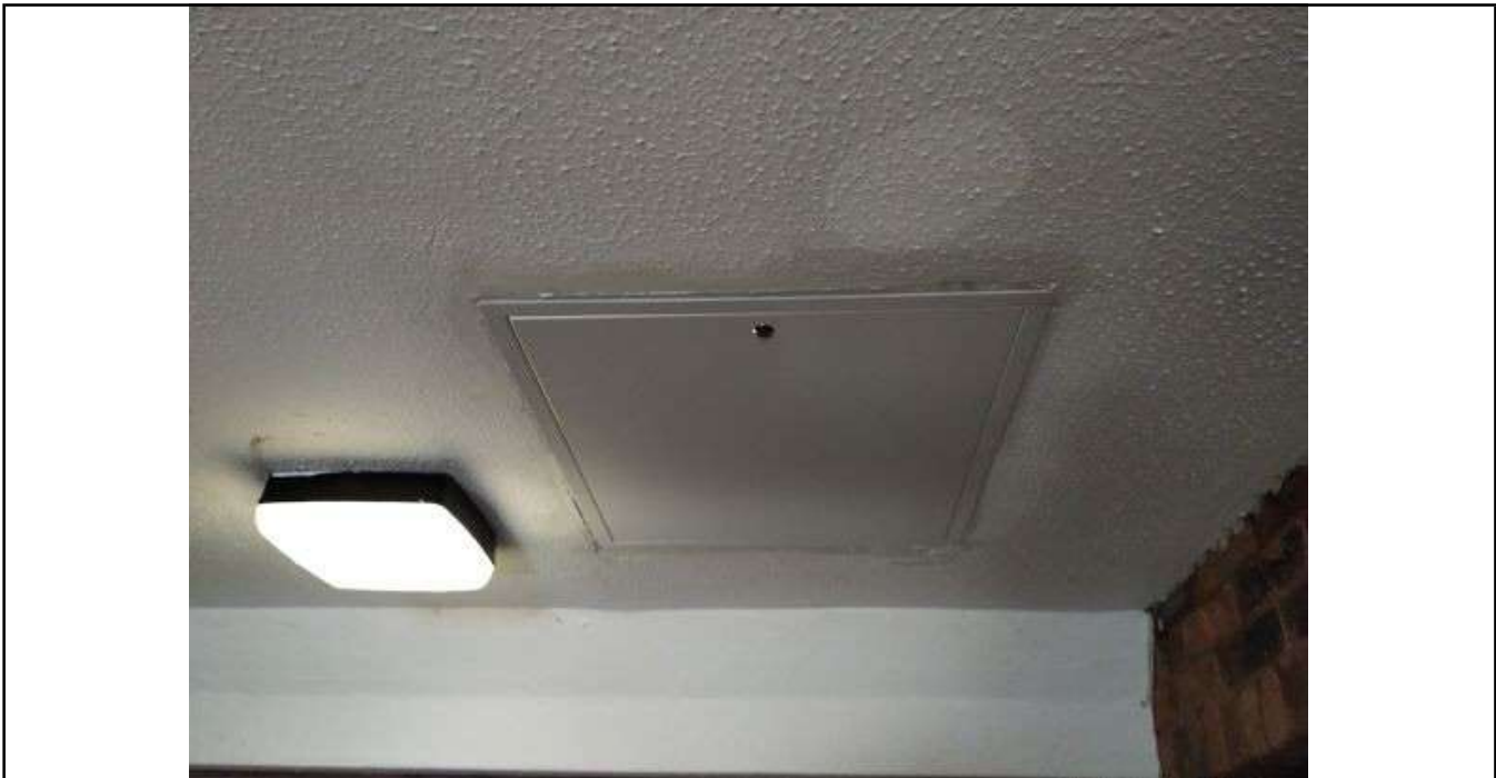
Photo No. 6 One Hour Fire Resisting loft hatch replaced after 2023 FRA.
