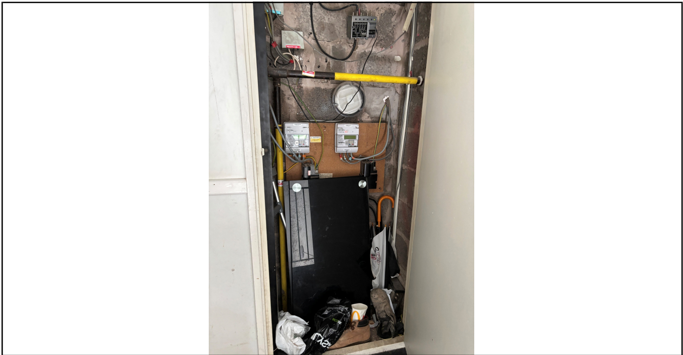
Photo No. 2 Personal items in service cupboard adjacent to Flats e and f
