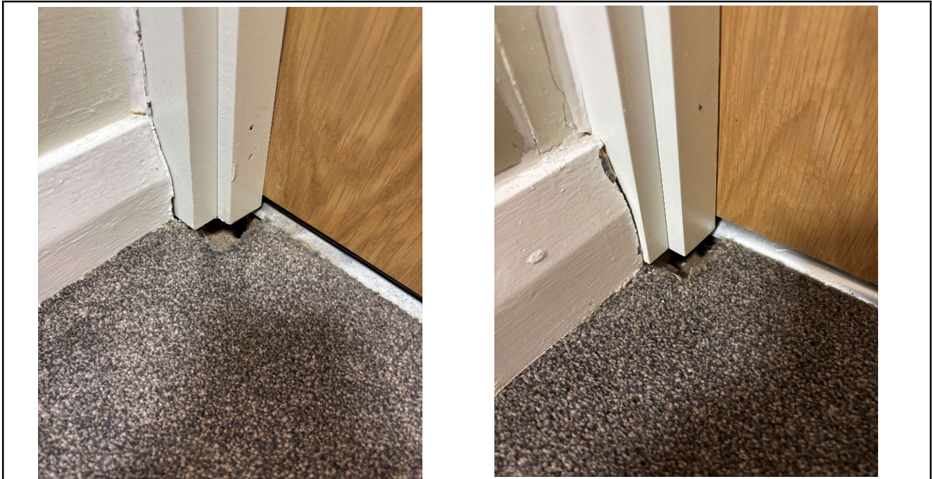
Photo No. 3 Examples of gaps under flat front door casings listed in 13.1
