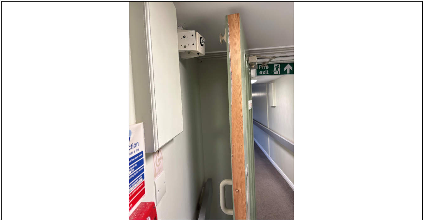
Photo No. 7 Corridor door nr Flat 20 Catching on carpet
