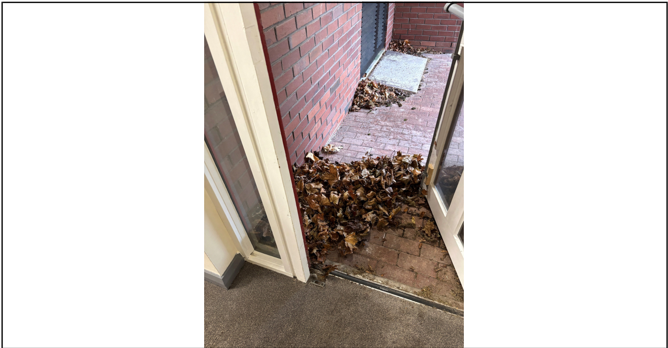
Photo No. 8 Leaves outside fire exit
