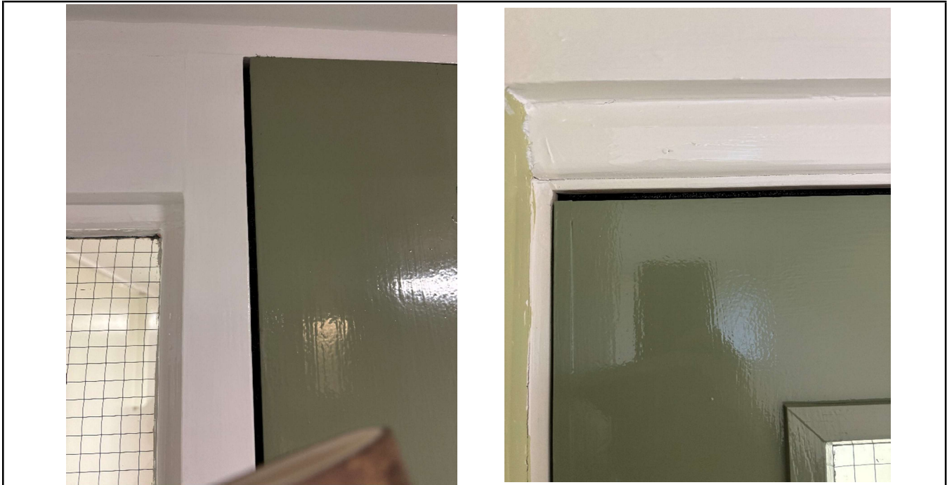
Photo No. 1 Example of excess gaps on fire doors listed in 12.1
