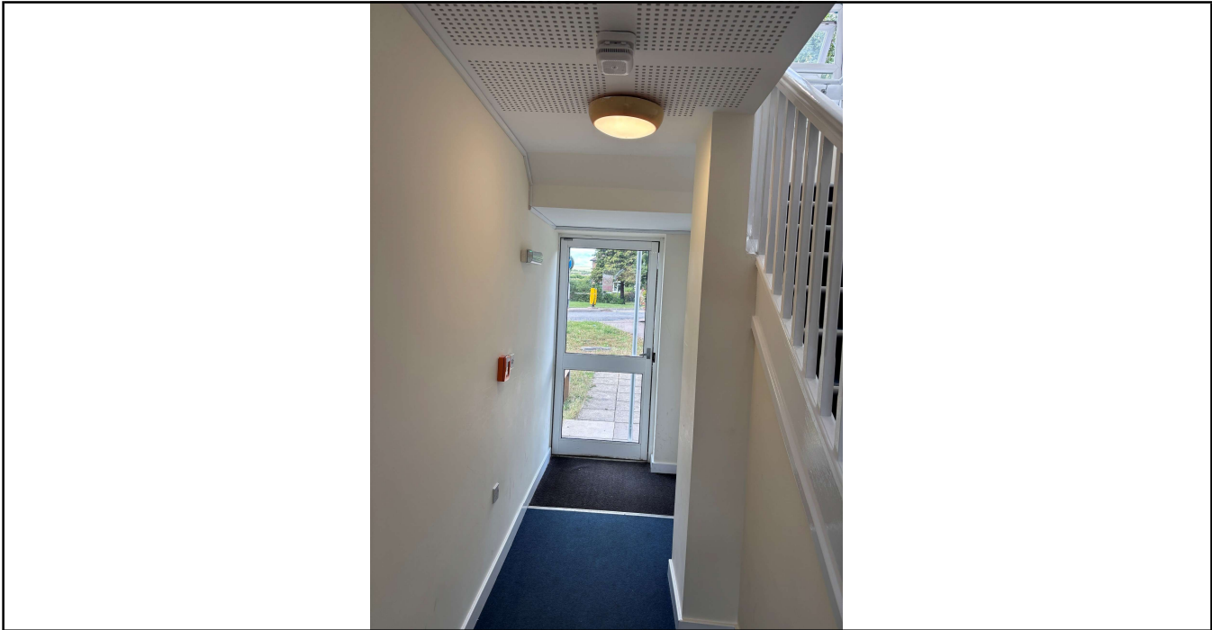
Photo No. 2 Rear Door View to main entrance AOV Point to the left. New Fire routine Notice installed.
