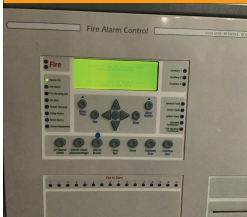
Fire alarm control panel
