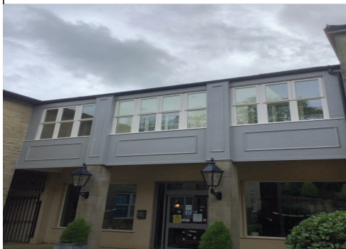
9.Unconfirmed cladding requires investigation to combustibility
