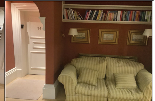
4.combustible items stored at base of stairwell and outside apartment 34
