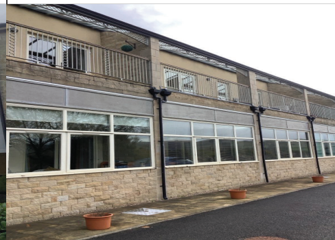
10.Unconfirmed cladding requires investigation to combustibility
