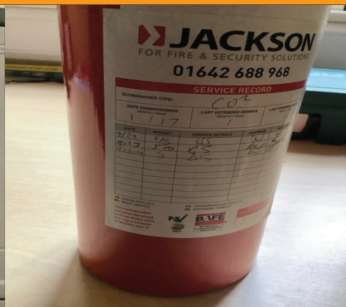
Fire extinguisher label
