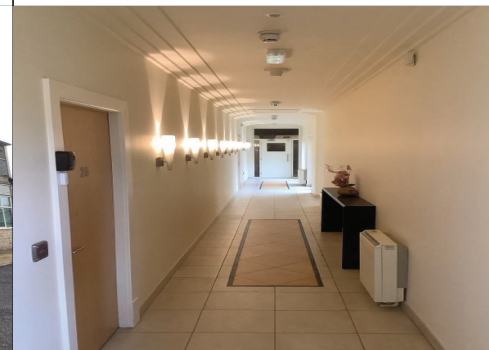
11.Direction exit signage required on corridor at Apt 26
