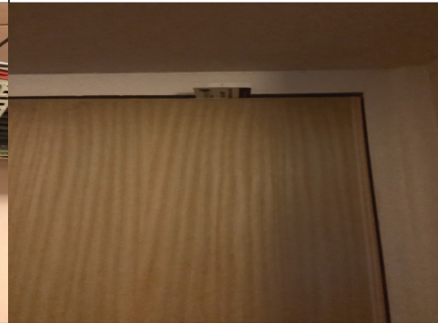
6.Flat26 has excessive gap at top of door. Reduce to 3mm
