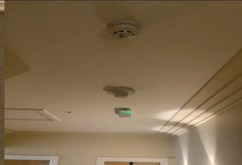
2.Emergency lighting and detection within communal areas of the corridors
