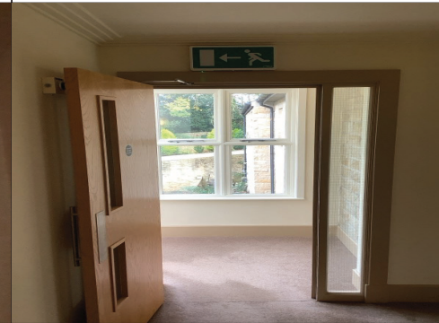
7.Direction exit sign pointing away from closest fire exit point on 1st floor
