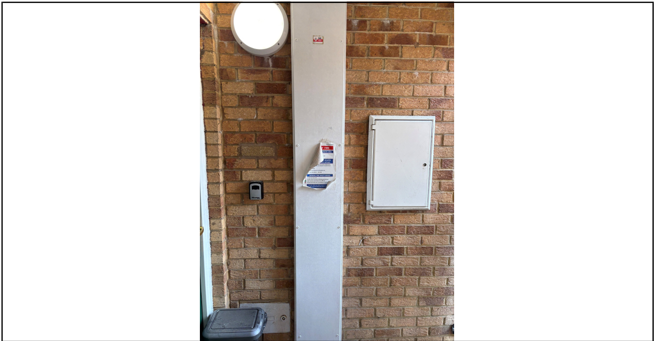
Photo No. 4 Evacuation notice damaged - Replaced
