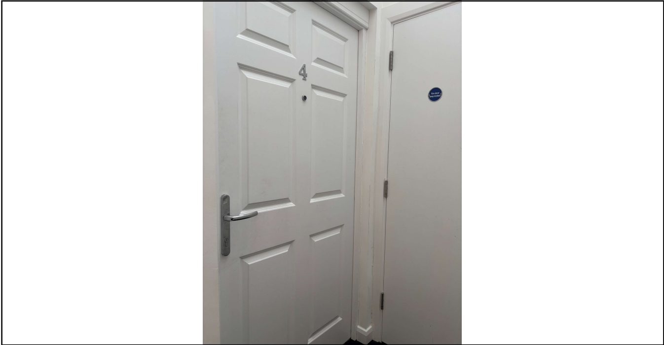
Photo No. 3 Head of Stairs no communal landing just left right.
