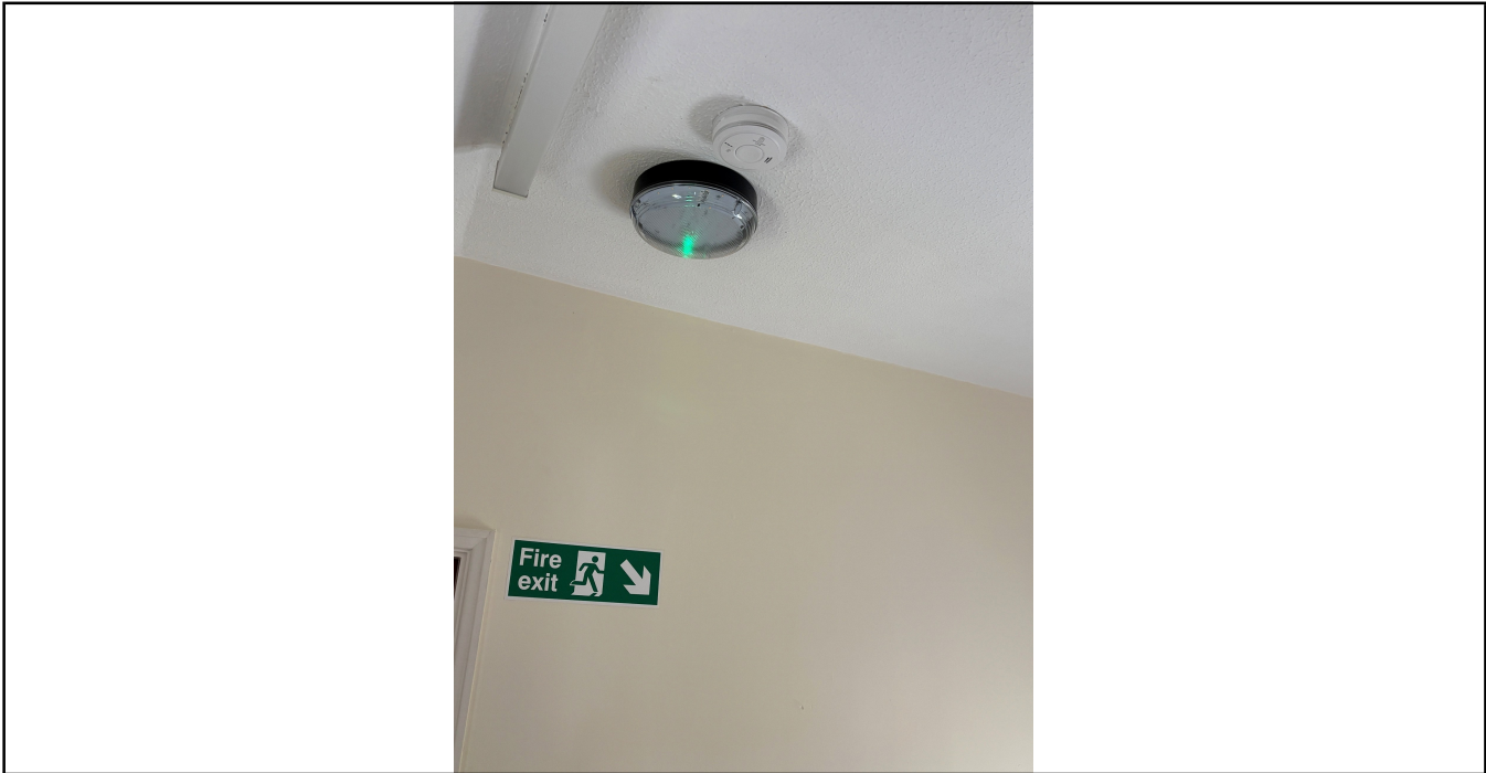
Photo No. 2 None Maintained EL and Directional Exit Signage.
