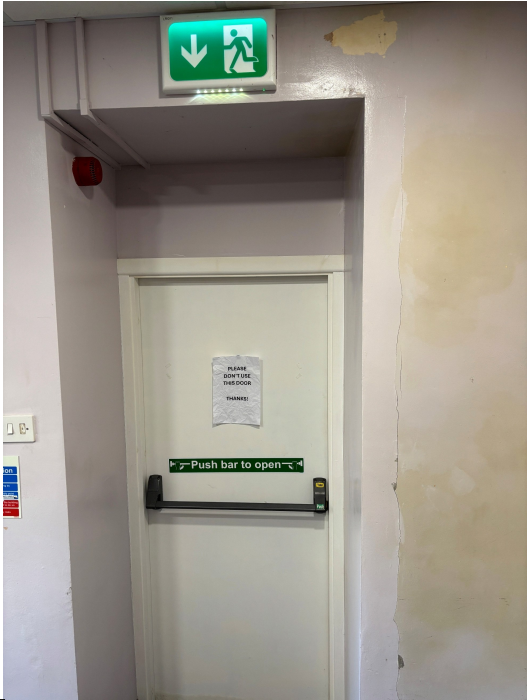
Photo No. 3 Notice on escape route 'please do not use this door'
