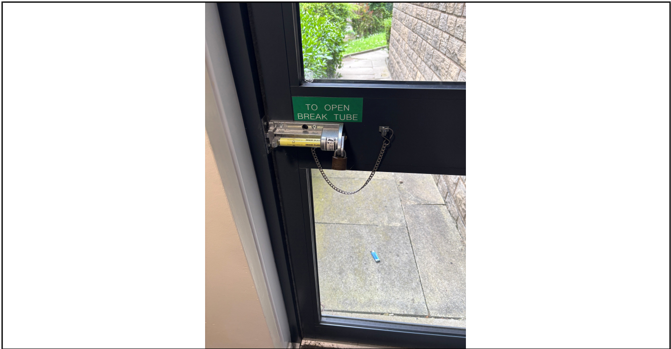
Photo No. 7 Hammer missing from break glass bolt
