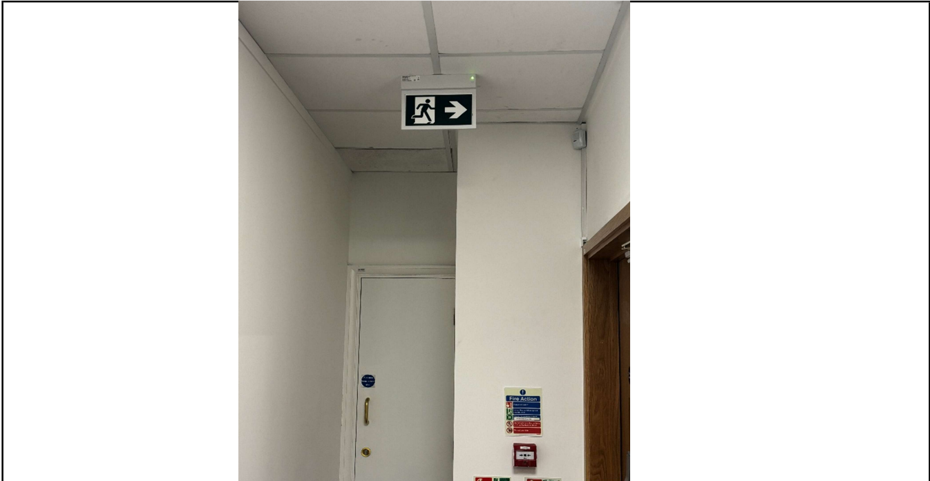
Photo No. 11 Non-Maintained Emergency Lighting Directional sign
