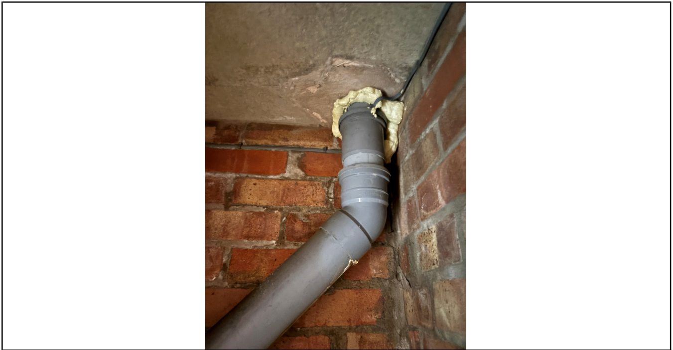
Photo No. 5 Compartmentation breaches filled with yellow foam 1st Floor
