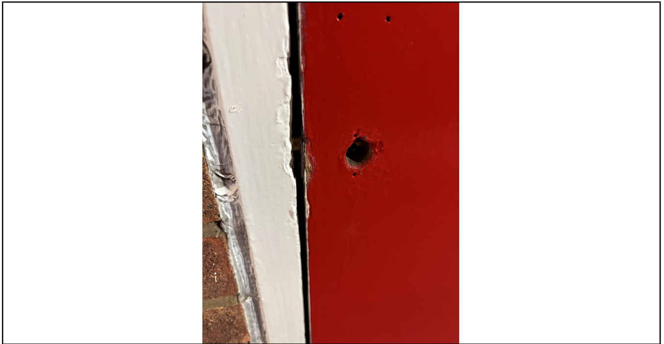
Photo No. 11 Electrical room door, unsuitable lock and damage 2nd F
