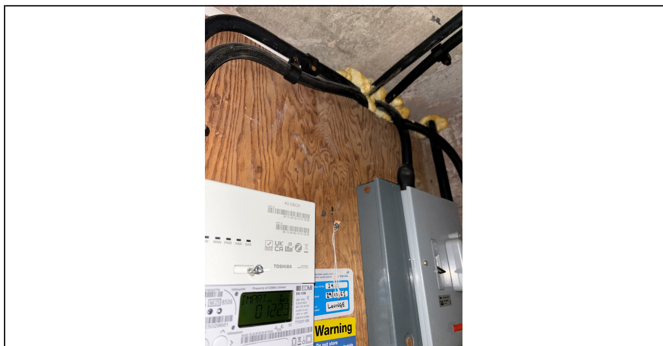
Photo No. 4 Compartmentation breaches filled with yellow foam 1st Floor
