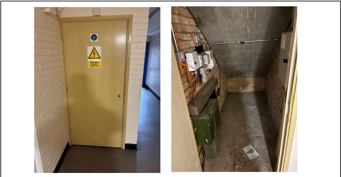
Photo No. 4 Electrical intake cupboard clear at the time of the audit.
