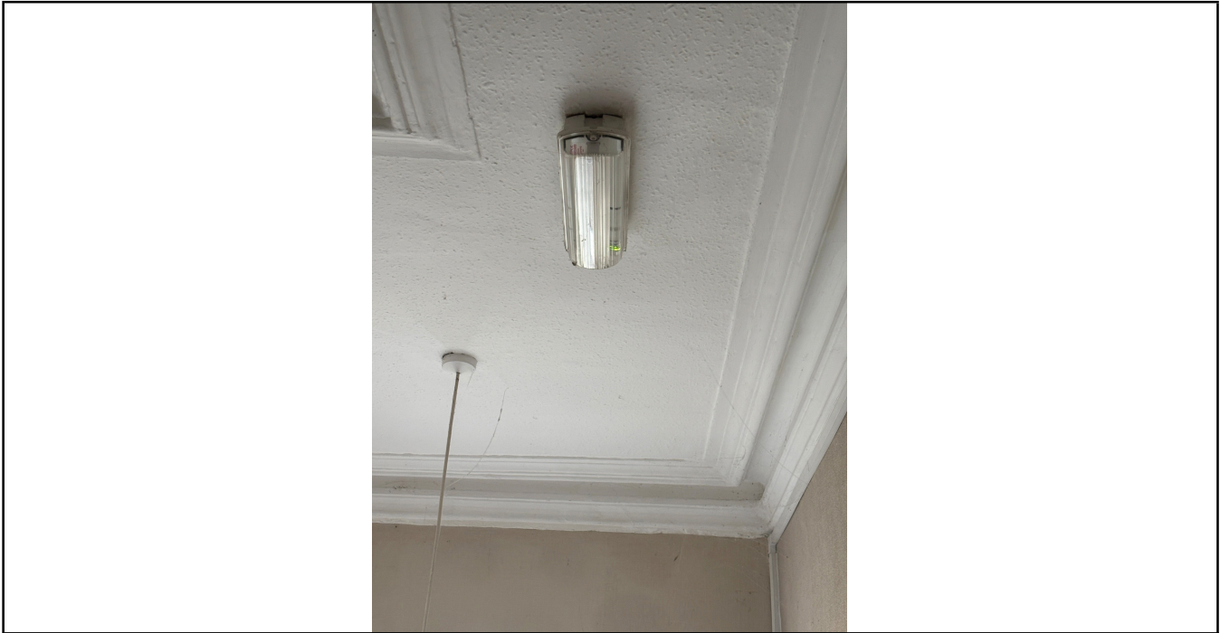
Photo No. 7 Non-Maintained Emergency Lighting.
