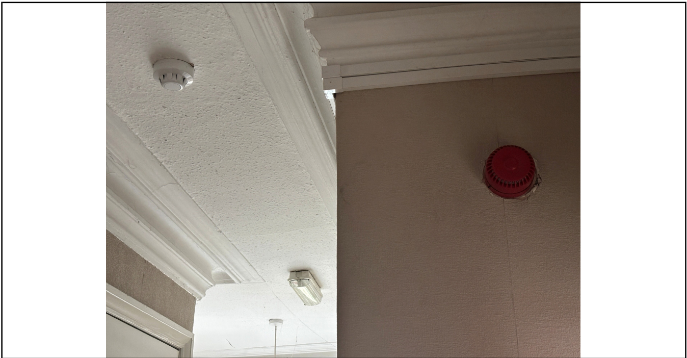
Photo No. 8 Detection and Sounders throughout the building. Sounders in every room.
