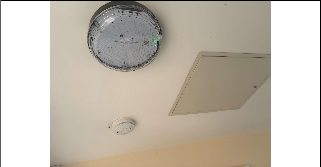
Photo No. 5 Second Floor Non maintained lights and loft hatch.
