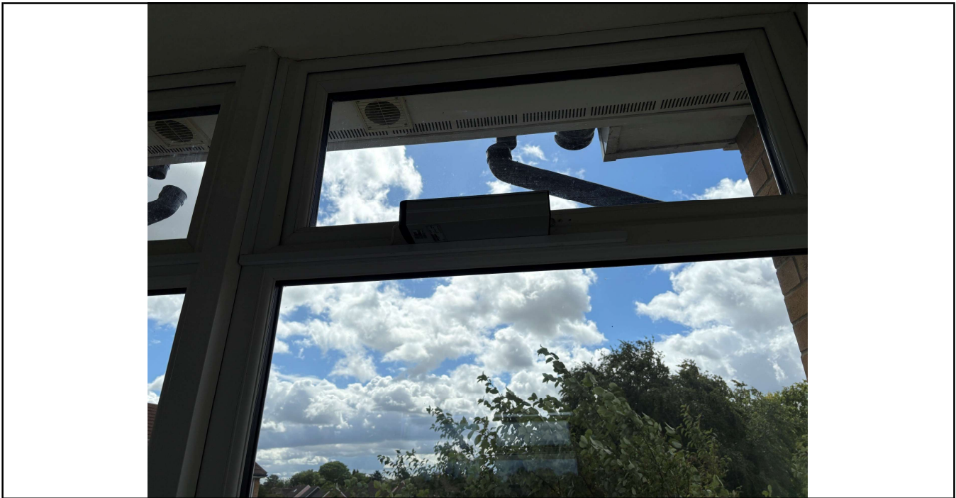
Photo No. 6 AOV acuaturs top floor functioning on day of inspection.
