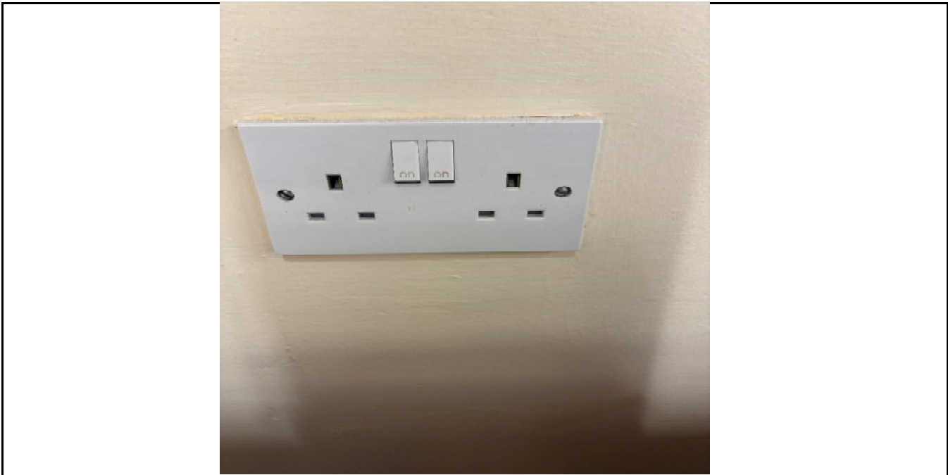
Photo No. 7 Electrical sockets and fittings in good condition
