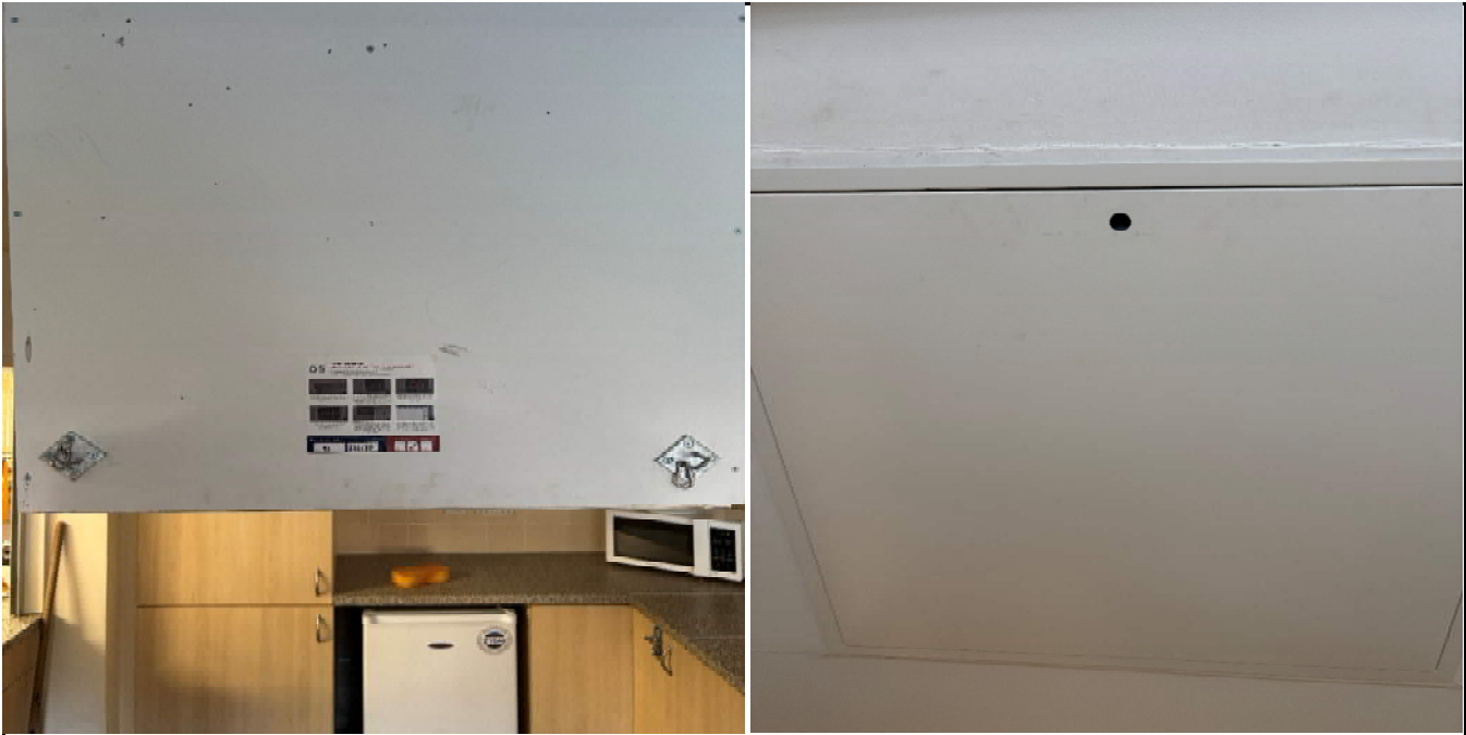
Photo No. 8 Fire retardant loft hatch
