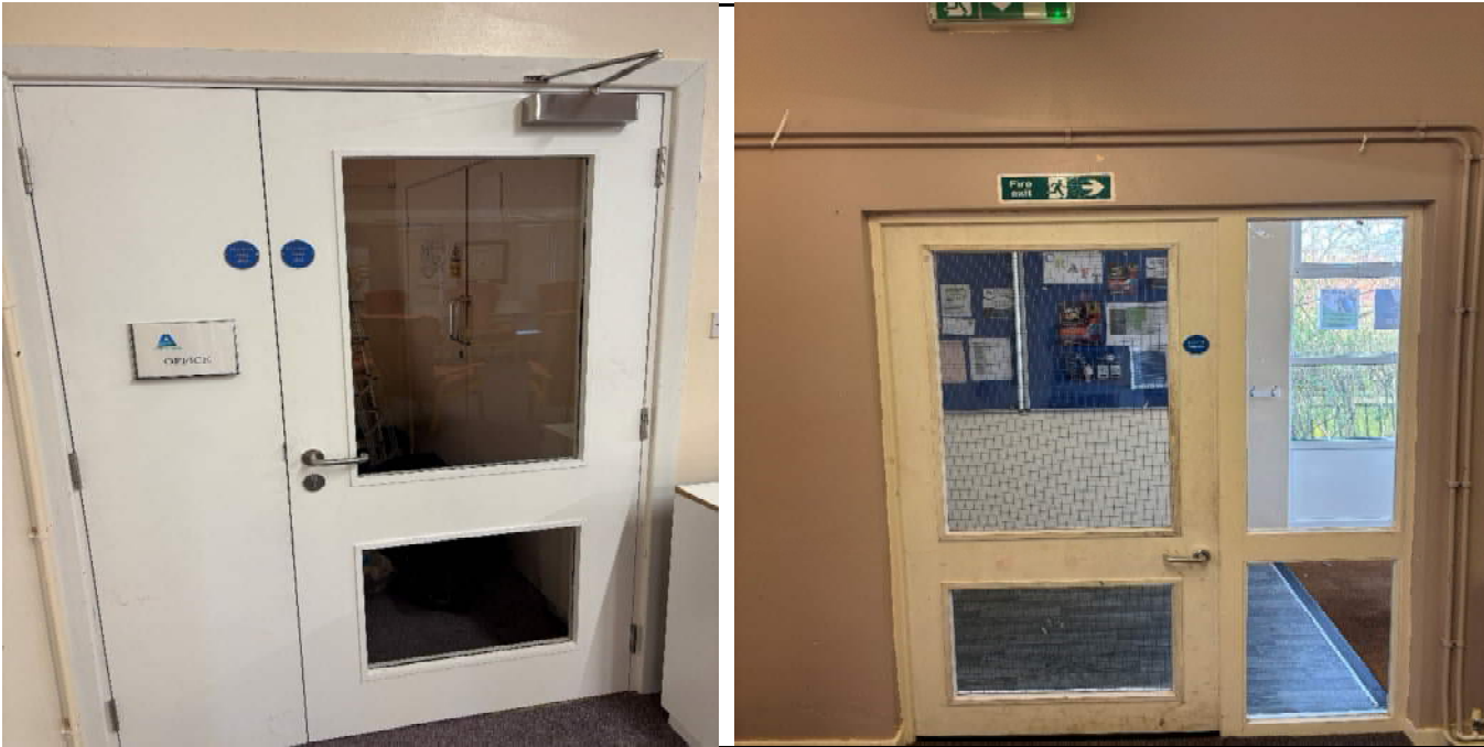
Photo No. 5 Typical internal fire door
