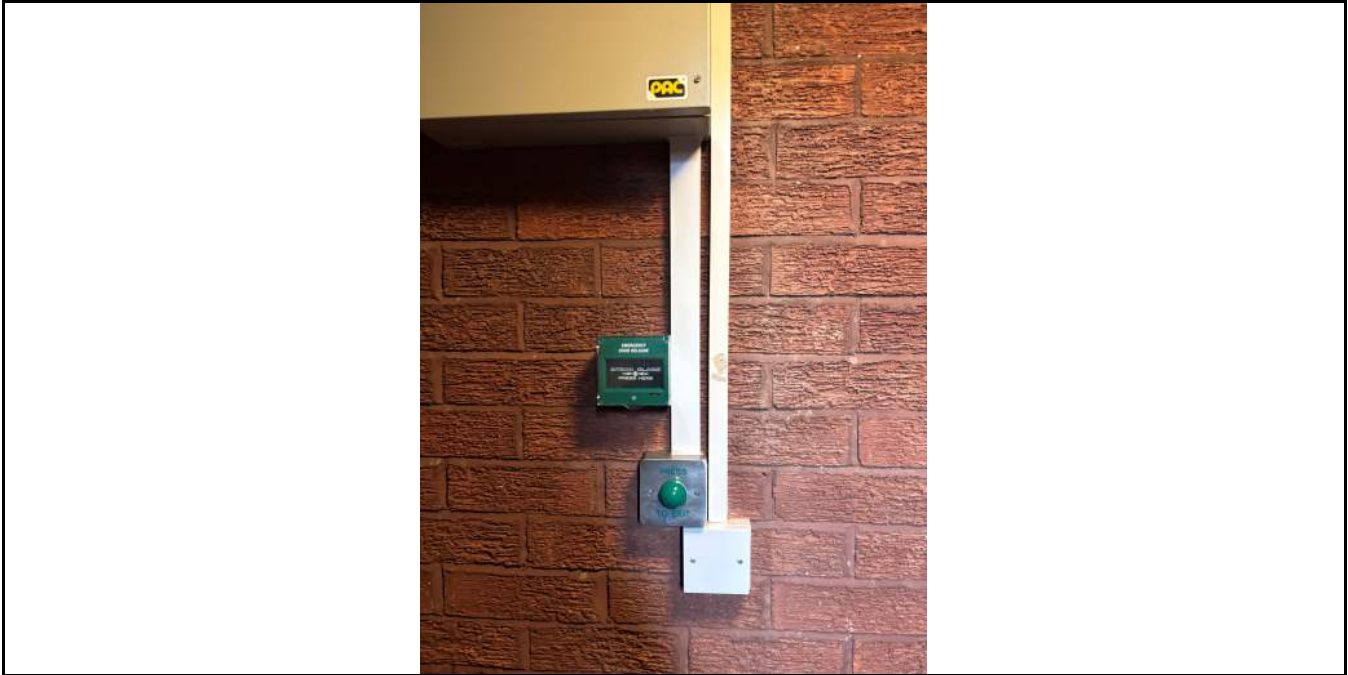
Photo No. 5 Push button and break glass exit button
