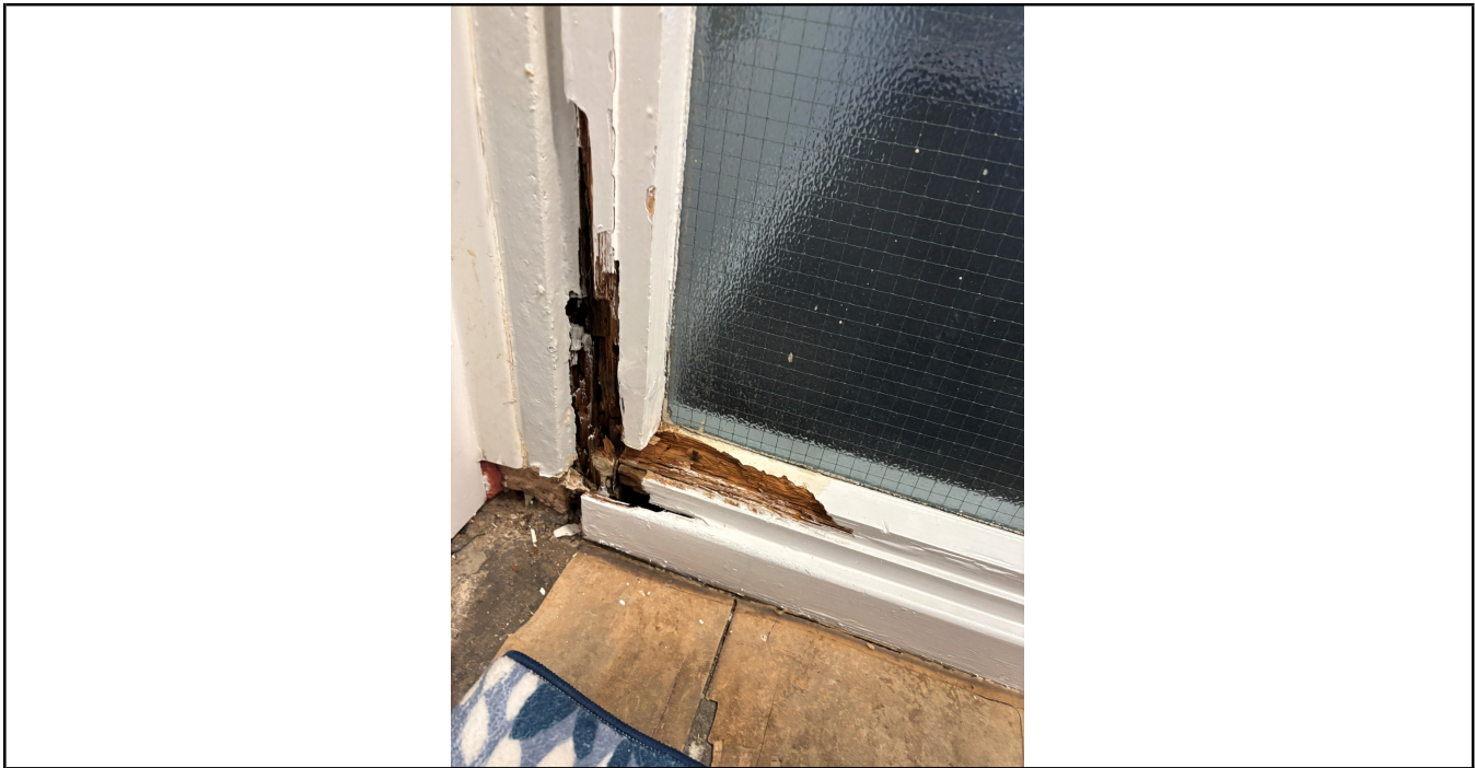
Photo No. 1 FR Lobby partition rotten in bottom corner nr Flats A & B
