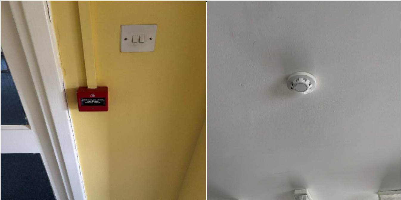
Photo No. 3 Fire detection and call points in good condition
