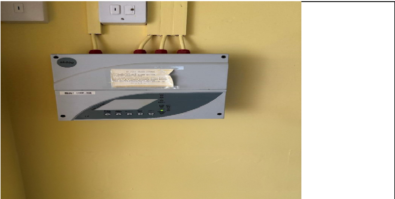
Photo No. 2 Fire panel
