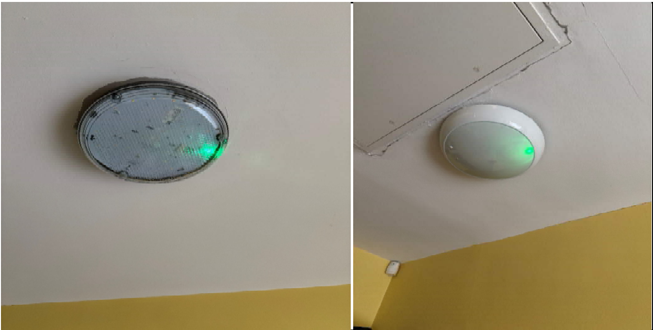
Photo No. 4 Emergency lights in good condition and secured
