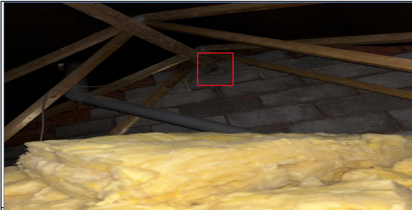
Photo No. 1 Compartmentation breach in roof space.
