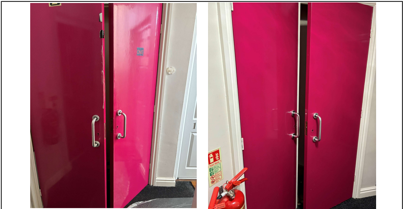
Photo No. 4 Communal store room doors unlocked and no signage.
