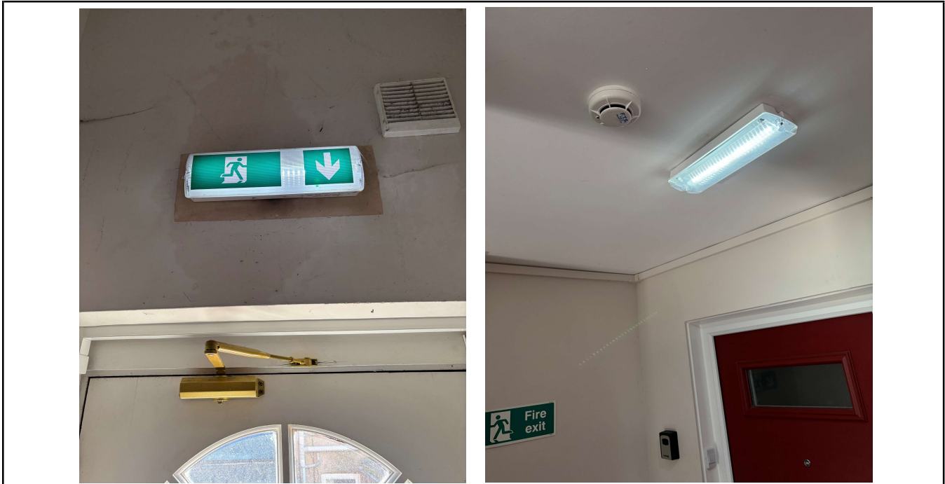
Photo No. 5 Emergency lighting and fire detection in communal areas
