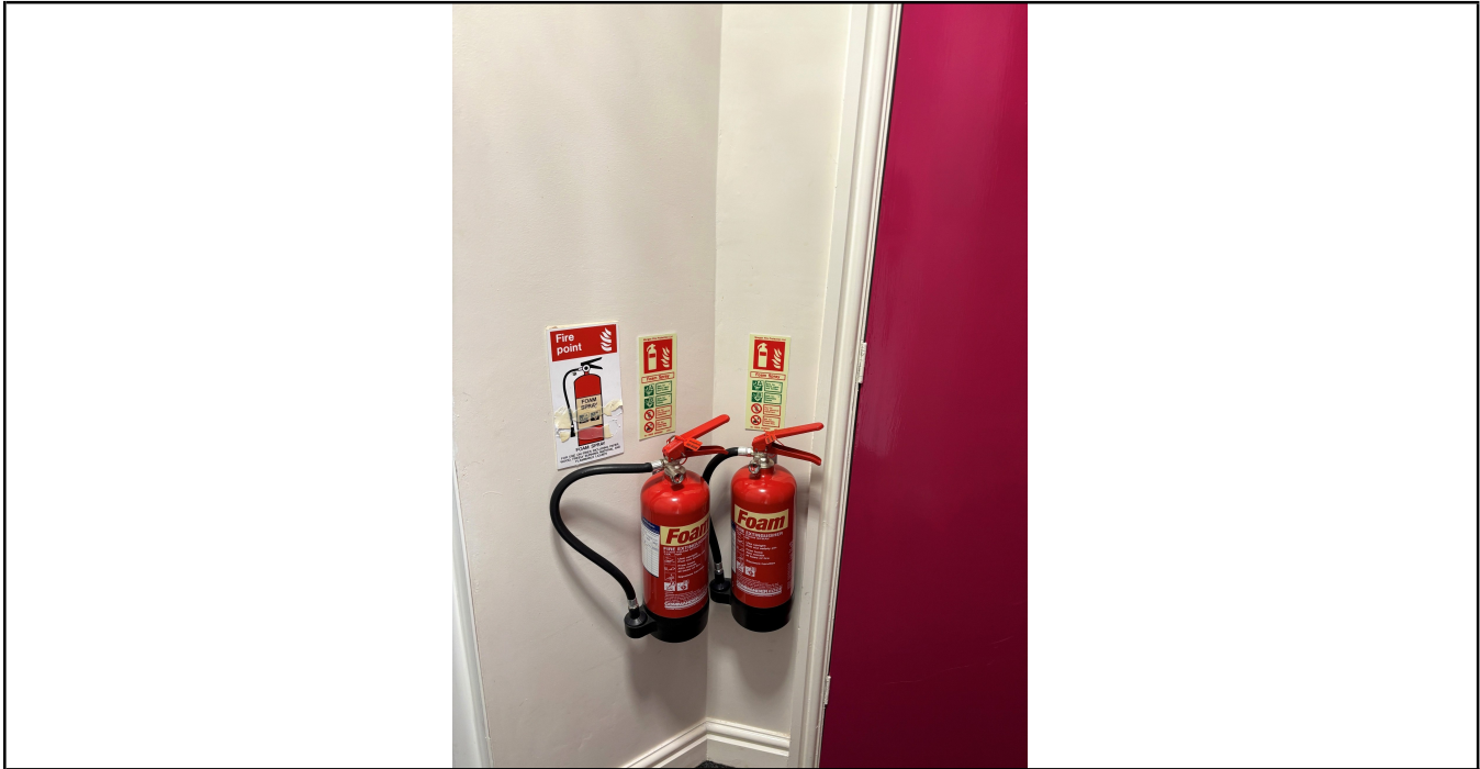
Photo No. 3 3 litre extinguishers provided on each landing
