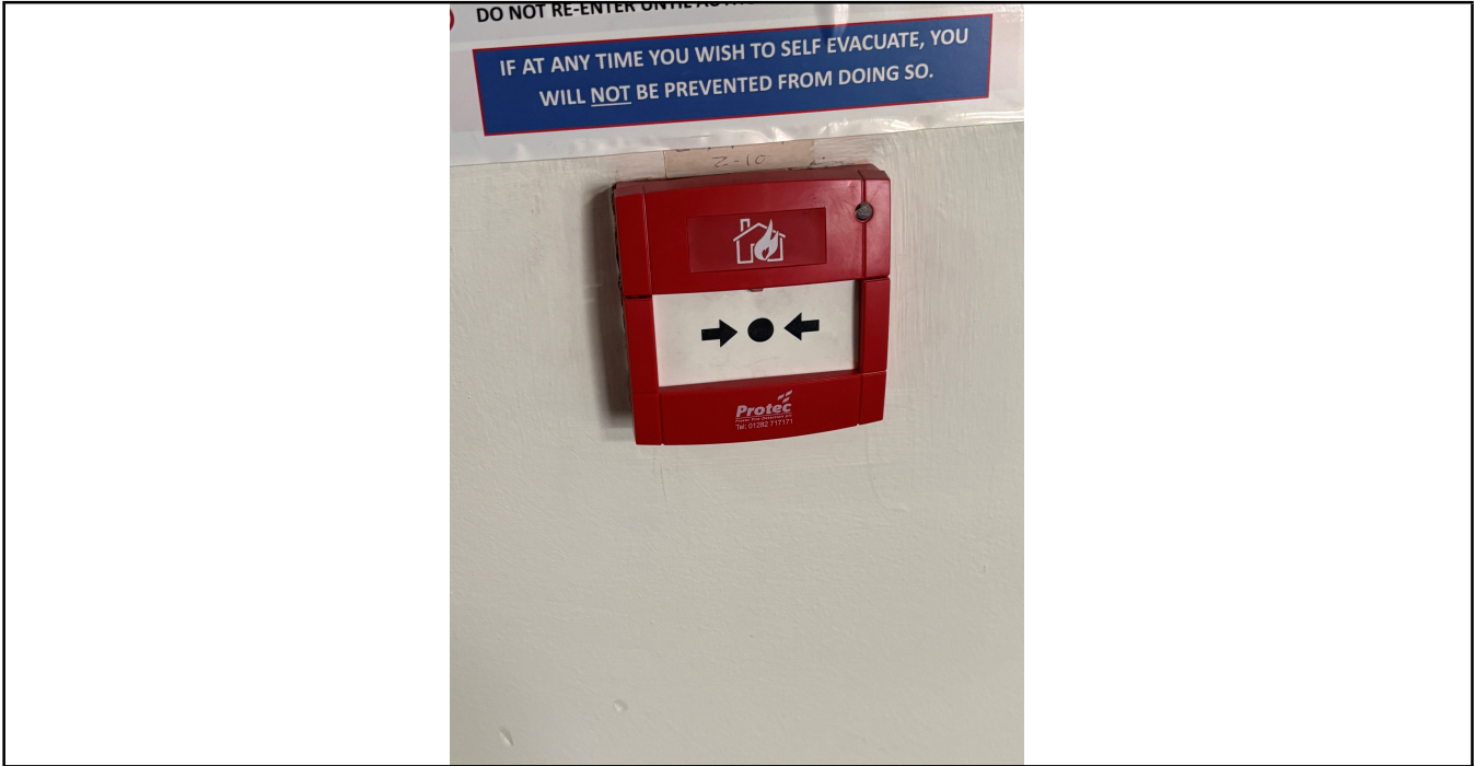
Photo No. 3 Shroud missing off all call points throughout the scheme
