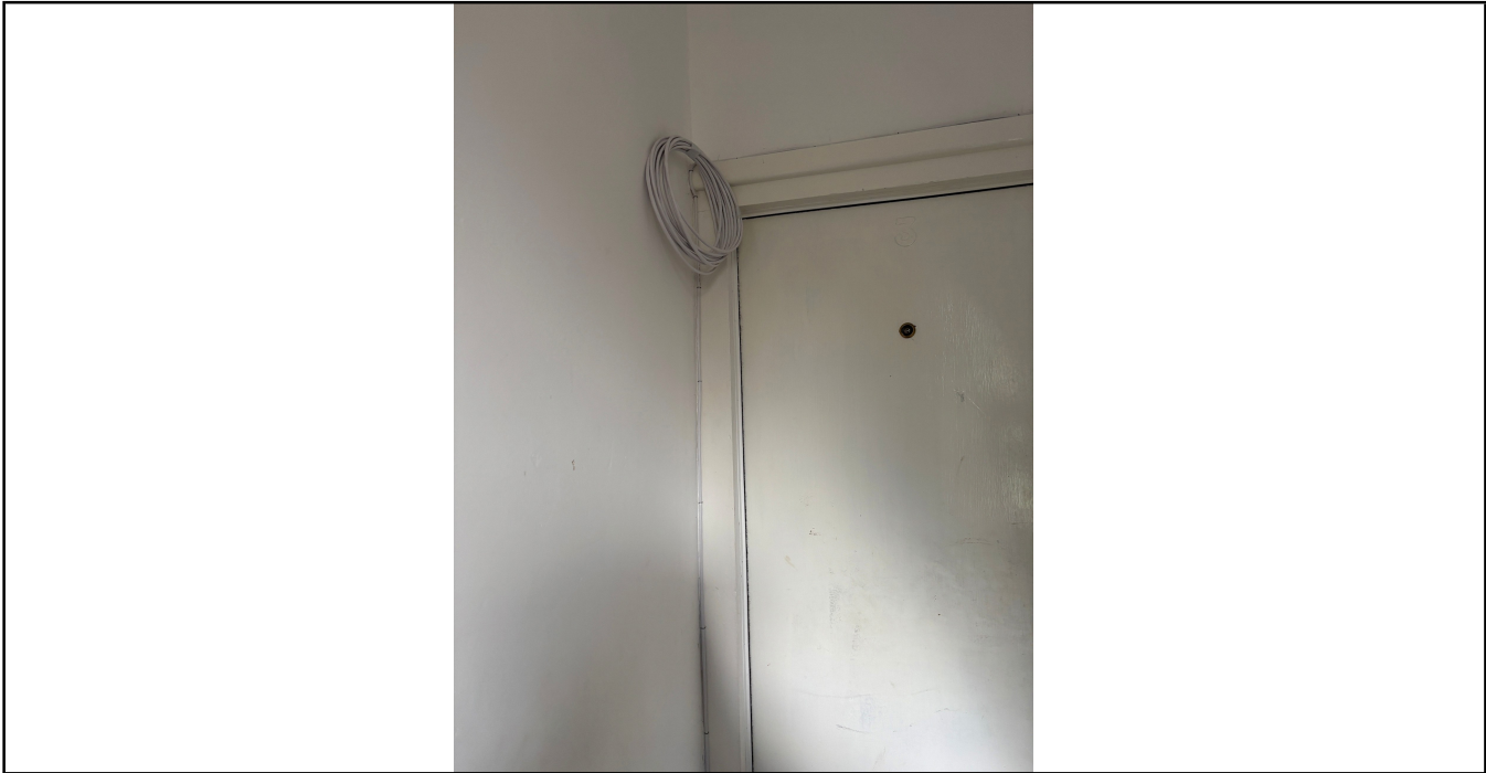
Photo No. 5 Coil of cable above Flat 3 door
