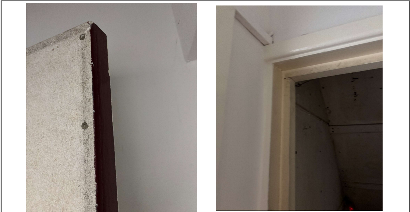
Photo No. 4 Basement door and frame hasn't got a combined seal fitted.
