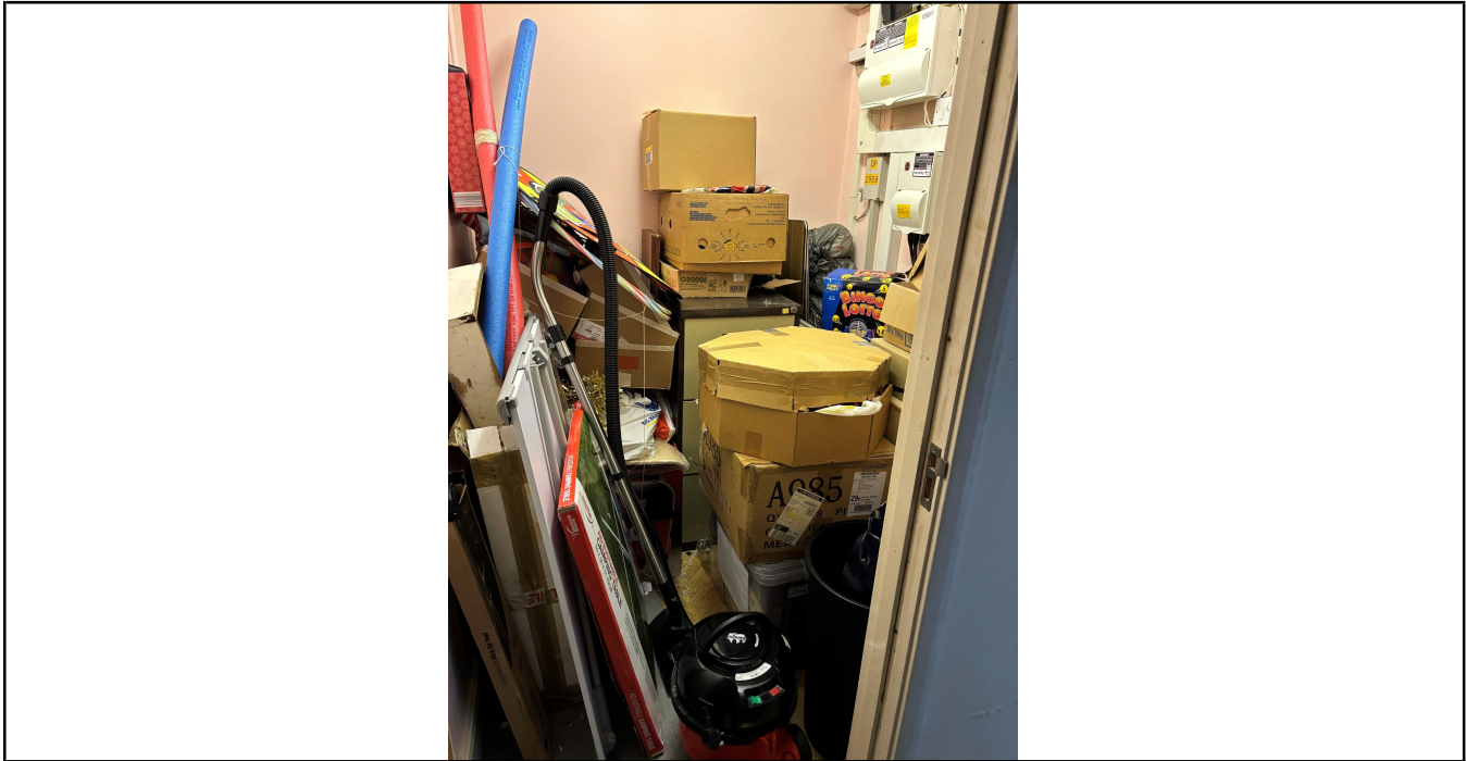
Photo No. 1 Store cupboard/electrical intake excess flammable storage
