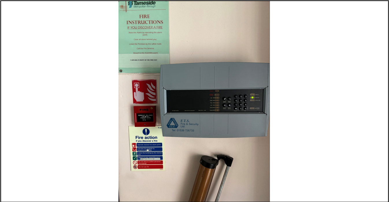
Photo No. 5 Fire alarm panel no faults
