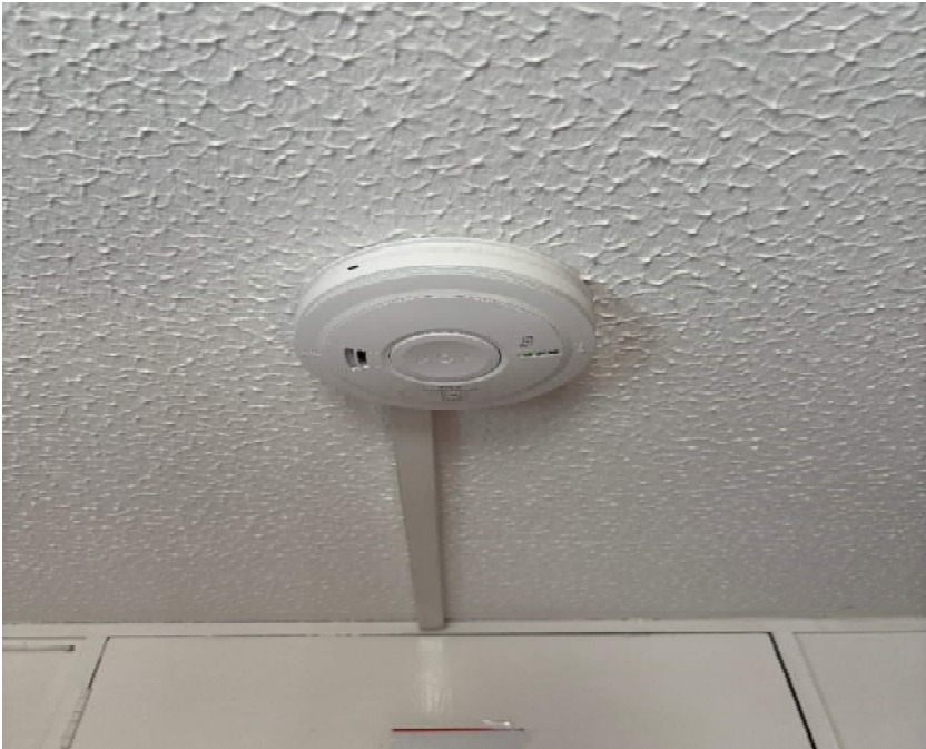
Photo No. 1 Fire detection fitted and in good condition
