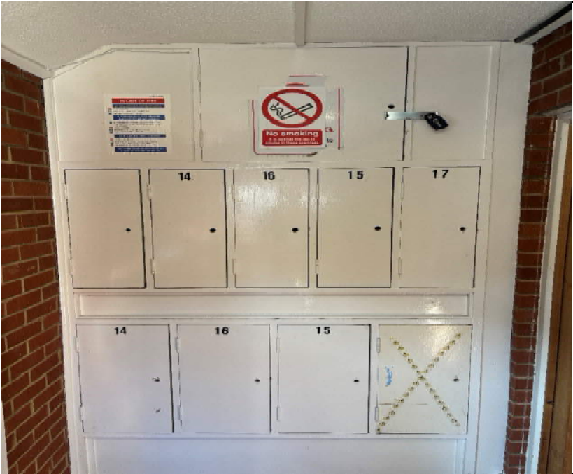
Photo No. 2 Electrical and gas intake cupboards with correct signage displayed
