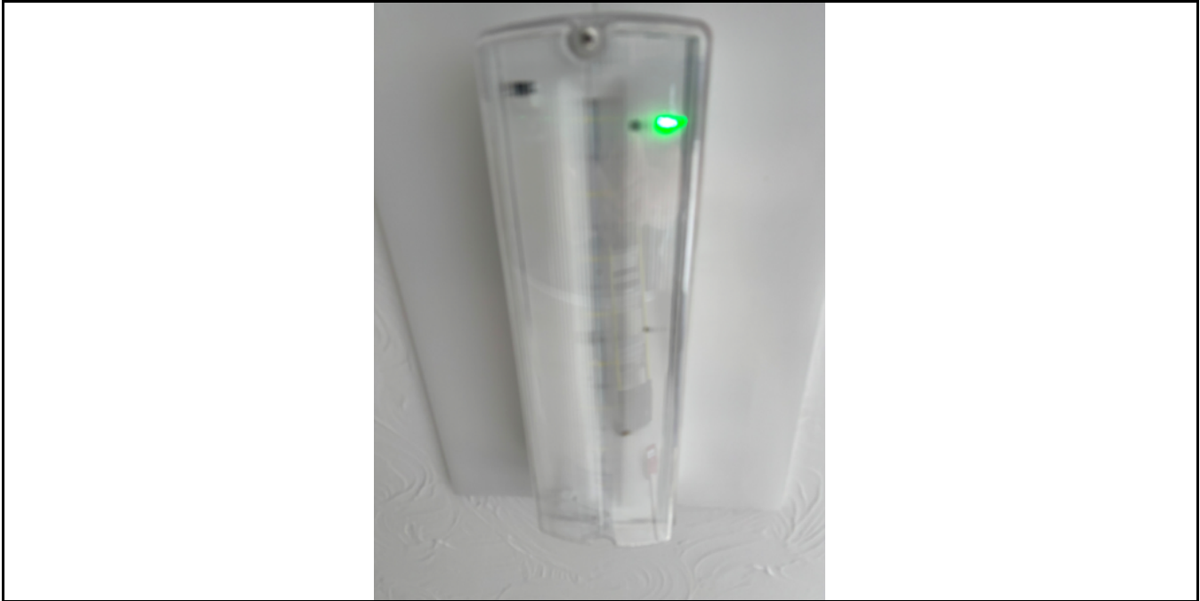
Photo No. 3 Emergency lights in good condition
