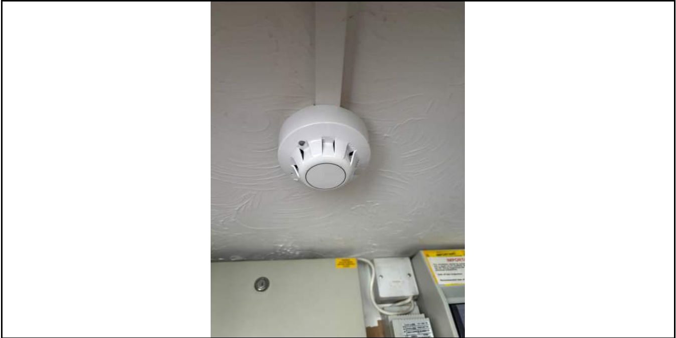
Photo No. 9 Detectors in electrical intake cupboard
