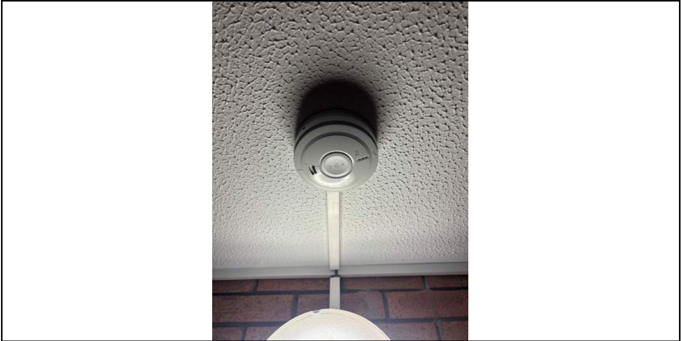
Photo No. 5 Communal fire detection head.
