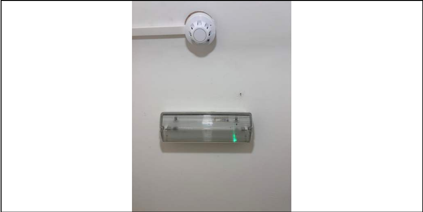
Photo No. 3 Emergency light and detector in good condition and secured
